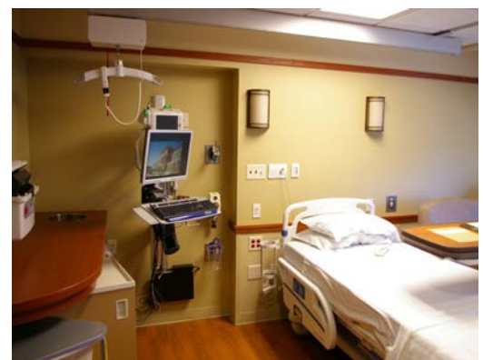
Figure 4.10.13: Nurse station in inpatient room. Elmhurst Memorial Hospital. Elmhurst, Illinois.
