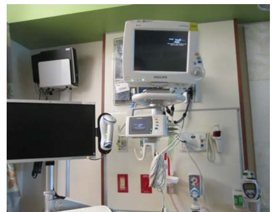
Figure 3.7.2: Controls surrounding patient bed. Lurie Children’s Hospital. Chicago, Illinois.
