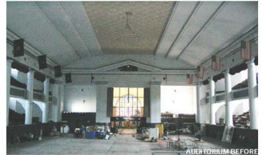
Figure C.1: A dropped ceiling erected in 1949 obscured the clerestory windows. Flood levels reached 18" above the auditorium floor of the building. Veterans Memorial Building. Cedar Rapids, Iowa.
