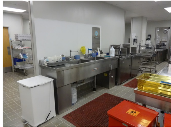
Figure 5: Decontamination Room (SPS)
