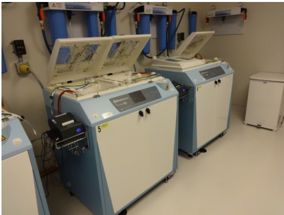
Figure 8: Scope Processing Room (SPS)
