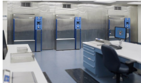
Figure 3: Steam Sterilization Room (SPS)
