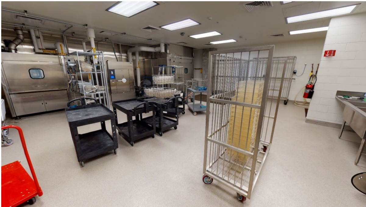
Image A.20 The Soiled Cage Room at the New Orleans VAMC R&D Facility contains dump stations, a bottle washer, a pass-through autoclave, a cage washer, and a rack which can be used to wash bottles and other equipment in the cage washer if the bottle washer is inoperable.
