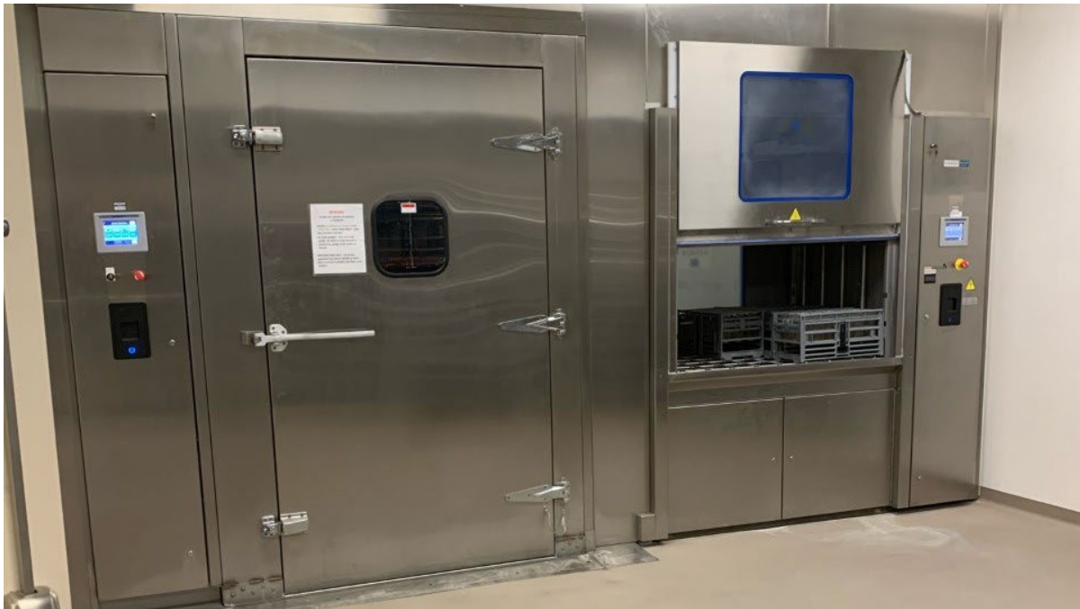
Image A.8 The Cagewash Area at the Rocky Mountain VAMC R&D Facility is separated into a clean side and a soiled side by the cage washer.
