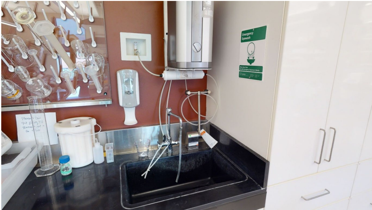
Image A.18 Every sink in the New Orleans VAMC R&D Facility laboratory includes a Safety Eyewash Station.
