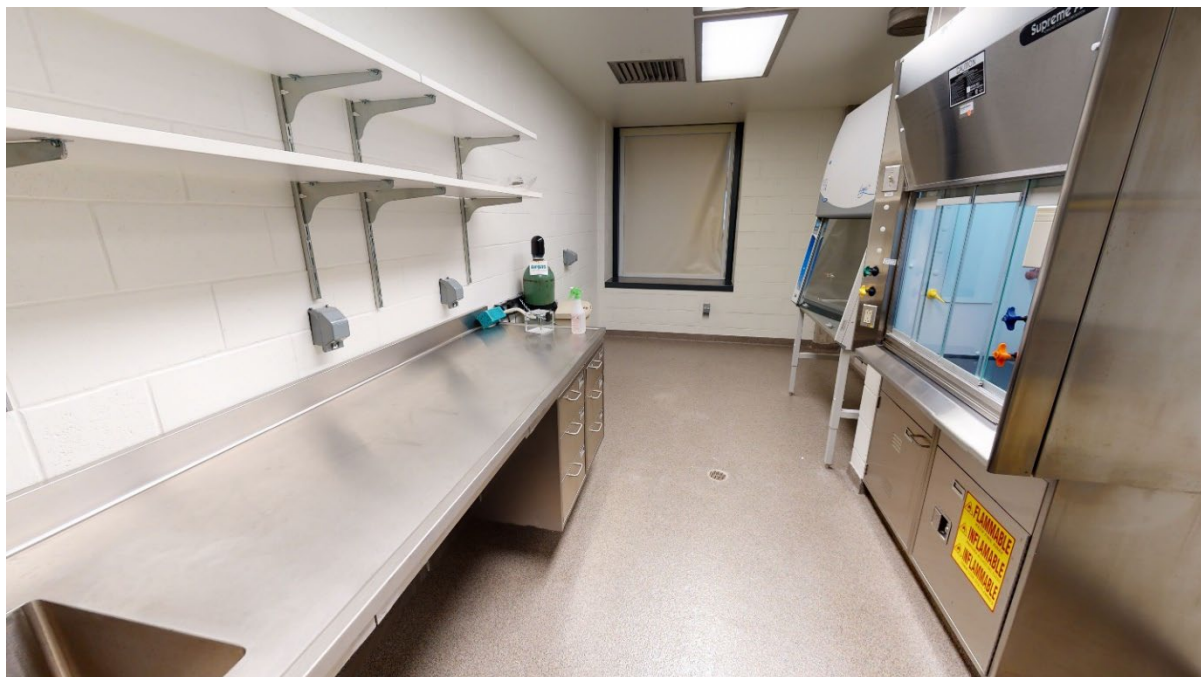
Image A.21 A VMU General Procedure / Treatment Room at the New Orleans VAMC R&D Facility contains stainless steel cabinetry, a biological safety cabinet, and a fume hood.
