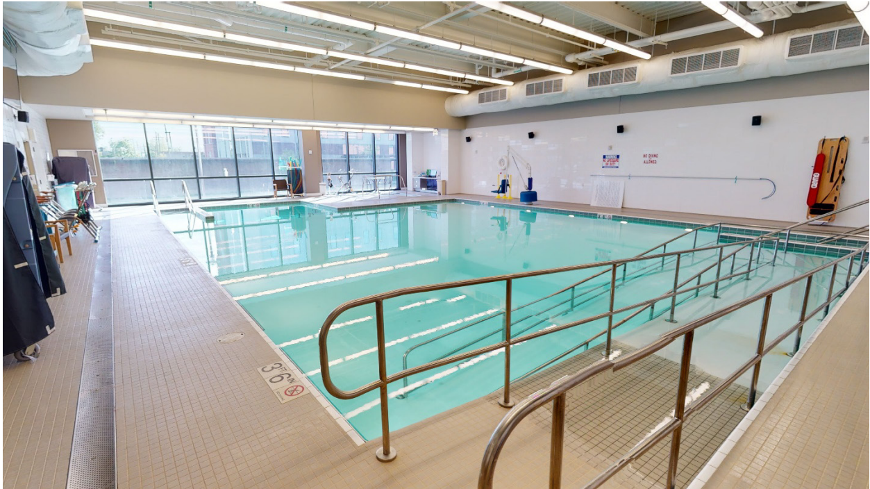
Figure 3.5 The Aquatic Therapy Pool at the New Orleans VAMC has a flat floor and is 3 feet, 6 inches deep. A deeper portion in the back is 8 feet deep.
