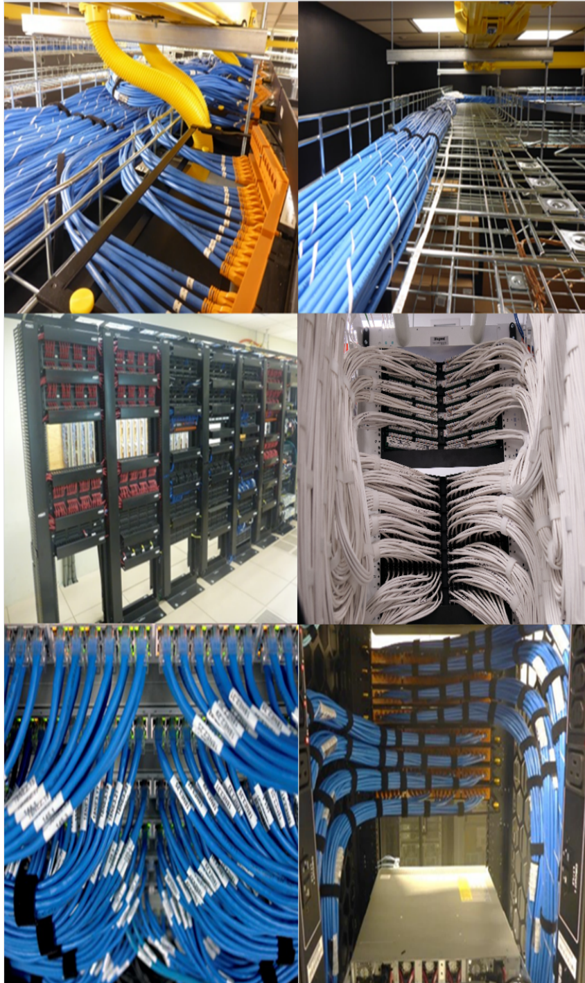
Figure 34: Acceptable Cable Management Results
