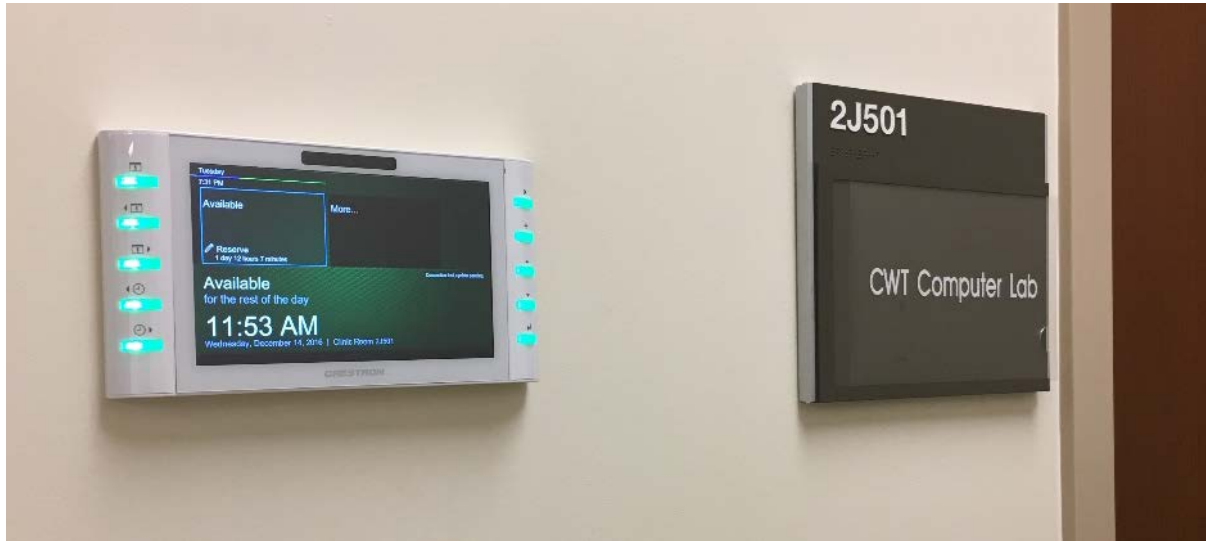
Figure 2.1.3.i. Electronic room scheduling display, Orlando VA Medical Center at Lake Nona
