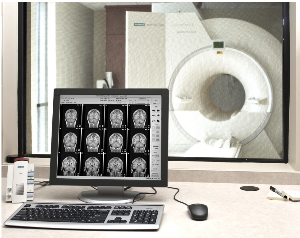
Figure 2.5.5.2: Example of a Control Room’s view to the imaging equipment. (Image used with permission from RAD-Planning)
