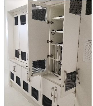
Technology storage in vented, but secure casework.
