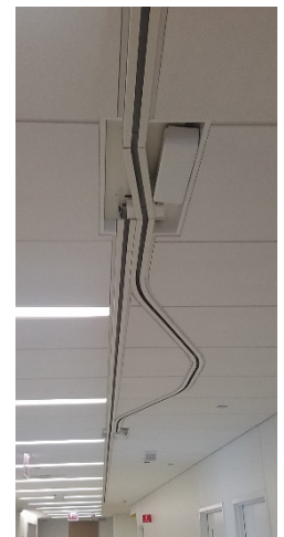
Overhead lift system
