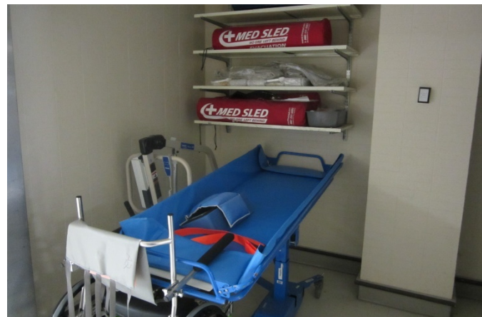
Life safety egress equipment including sleds
