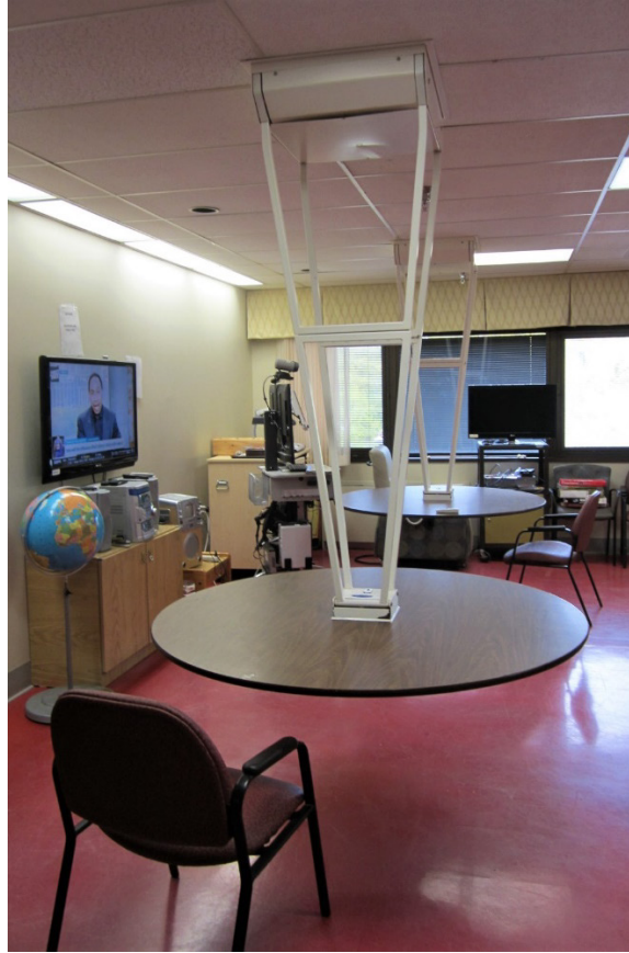
Figure 2.12 West Roxbury VAMC ceiling mounted retractable table installation
