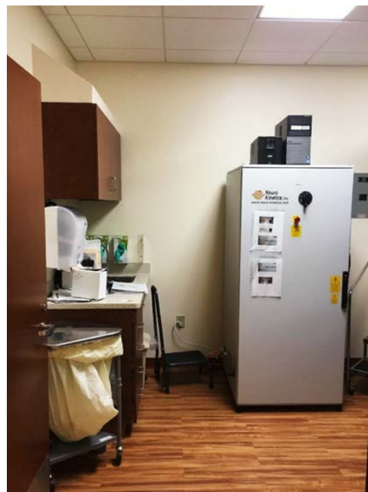
Figure 110: Rotary Chair Room: Electrical Console
