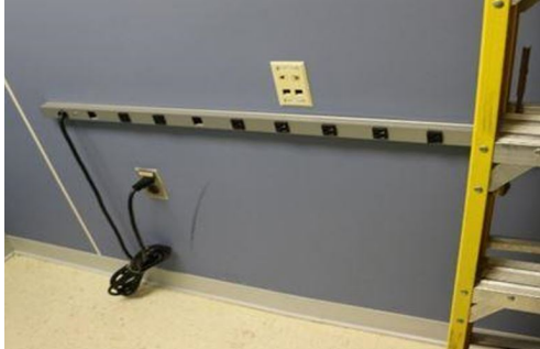
Figure 10 – power strip for SHM charging
