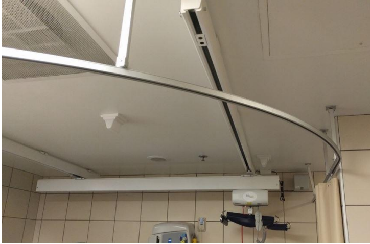
Figure 6 – lift rail above shower curtain rail minimizes interference
