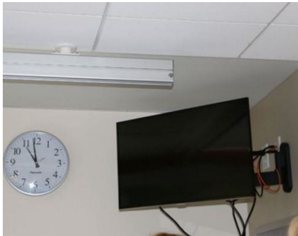
Figure 39 – monitor on wall mount
