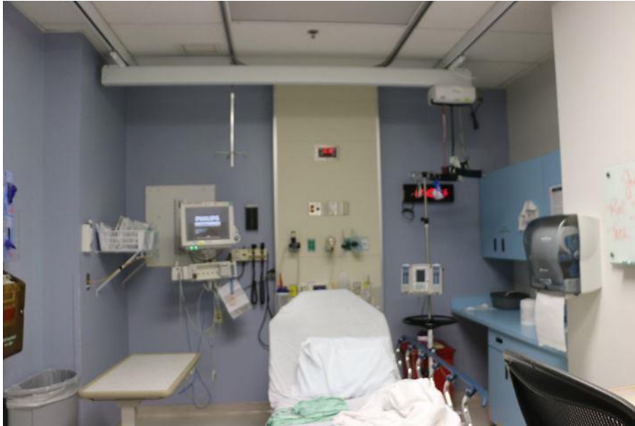
Figure 15 – traverse lift showing full room coverage at Emergency Department exam room
