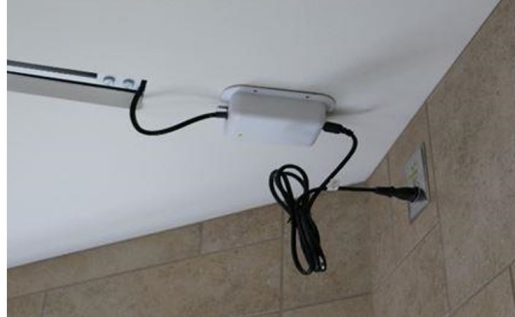
Figure 11 – outlet near ceiling for lift motor charging
