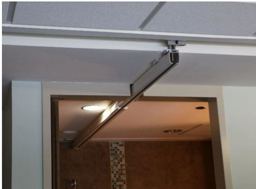
Figure 12 – door head gap for lift access to bathroom
