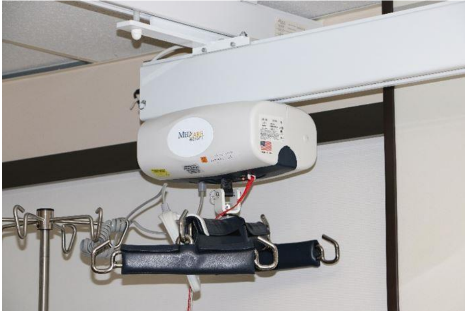
Figure 18 – potential conflict between carriage and top of IV stand
