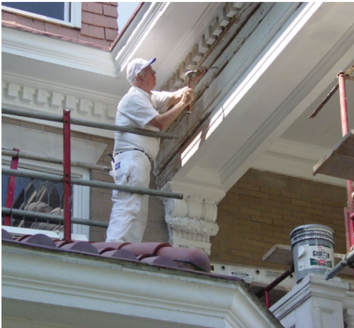
[12] Repair and limited replacement in kind to match deteriorated wood porch features is always a recommended preservation treatment.
