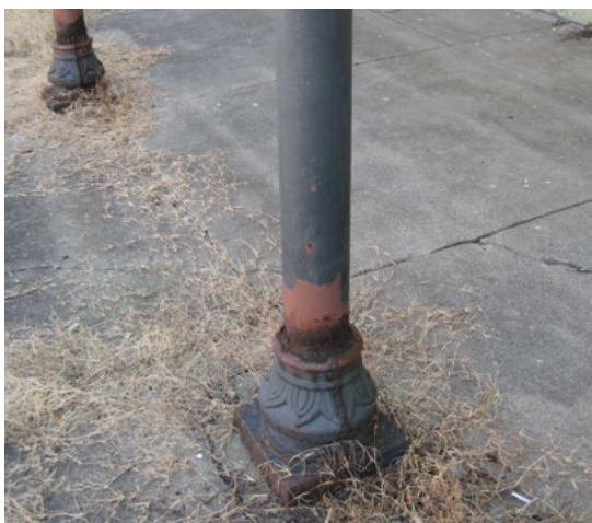
[7] (a) After the damaged portions of the base were repaired, (b) the cast-iron columns were cleaned and repainted to protect the metal from rusting.
