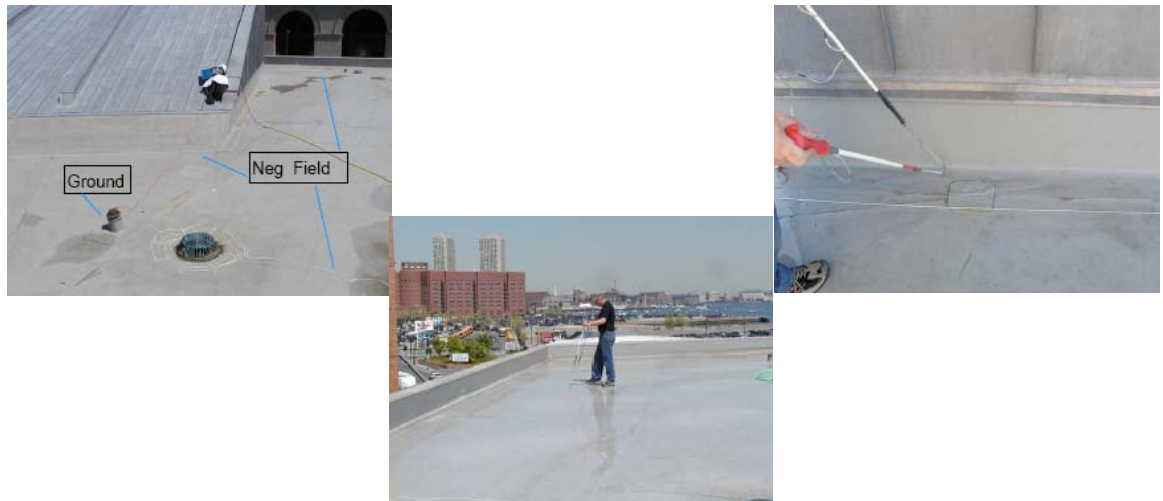
Figures 15 through 17 for roofing, waterproofing and vegetated roofs, Electric Field Vector Mapping is an extremely useful and accurate tool for pin-pointing leaks.
