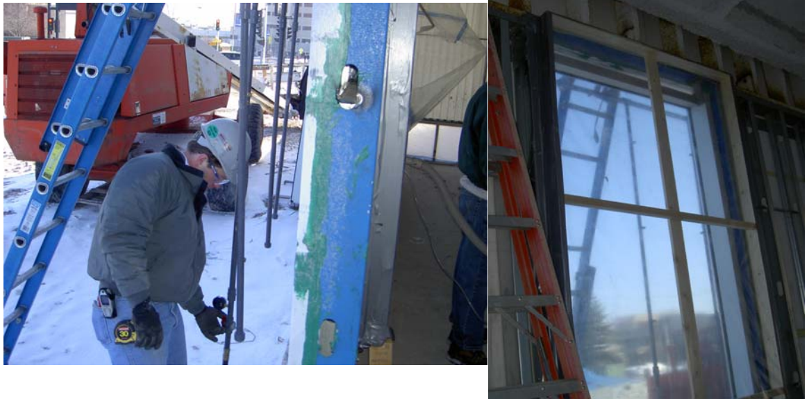
Figures 12 and 13: Field-testing of water penetration to ASTM E 1105 with spray rack.
