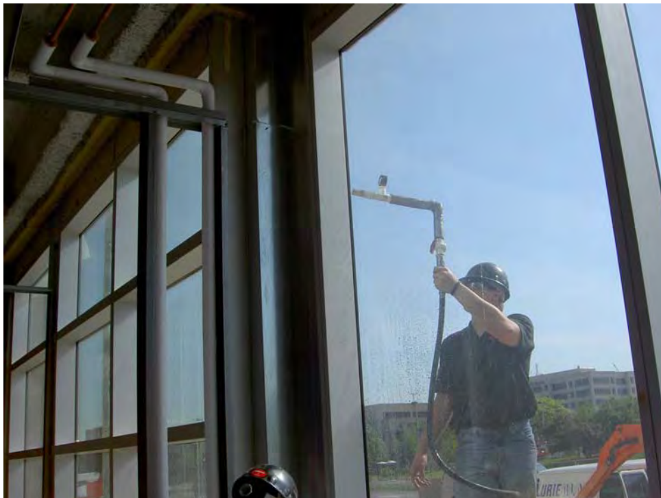
Figure 14 Hose spray testing at 15 psi, AAMA 501.2 test protocol. This is a simple test that discovers problems quickly
