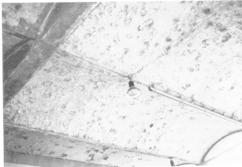
Ceiling of a gymnasium in a high school showing evidence of damage from basketballs thrown by students
