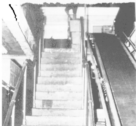
High activity level near friable asbestos
