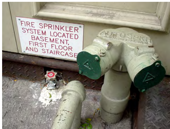
Figure 8.9. A sign indicating the areas covered by the sprinkler system that is fed by the FDC shown.
