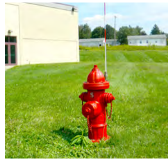
Figure 4.7. A dry barrel fire hydrant.
