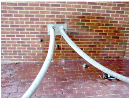
Figure 10.1. Charged hose lines connected to a wall-mounted FDC with two inlets.
