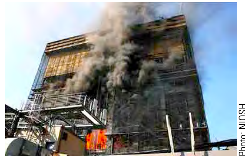
Figure 13.18. The fatal 2007 fire at New York City's Deutsche Bank Building.
