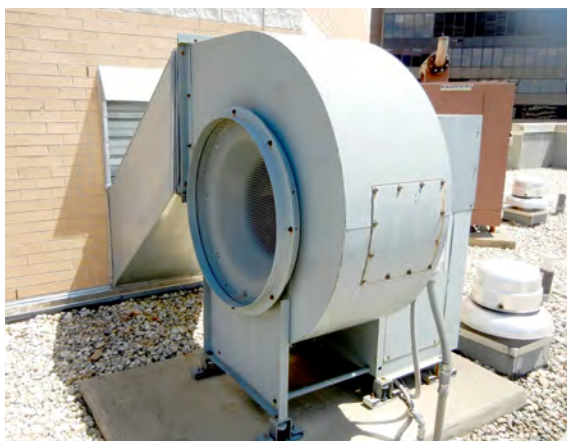
Figure 12.12. A stair pressurization fan.
