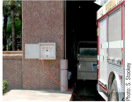
Figure 12.7. An exterior FDCP being supplied by a fire service mobile air unit.
