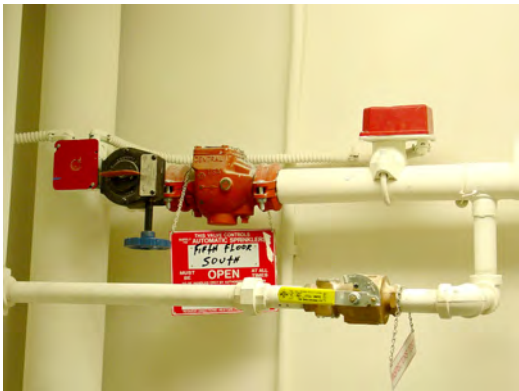
Figure 8.2. A sprinkler zone control station. The sign on the control valve indicates “first floor south” but there is no indication where the boundary is between south and north.
