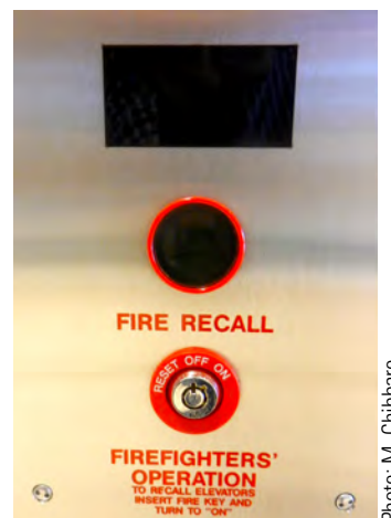
Figure 6.11. An elevator lobby switch for manual fire service recall.
