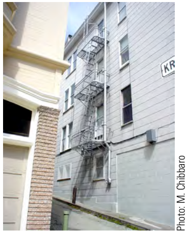
Figure 9.1. An exterior dry standpipe with an FDC on the bottom and a FHC at each fire escape platform.
