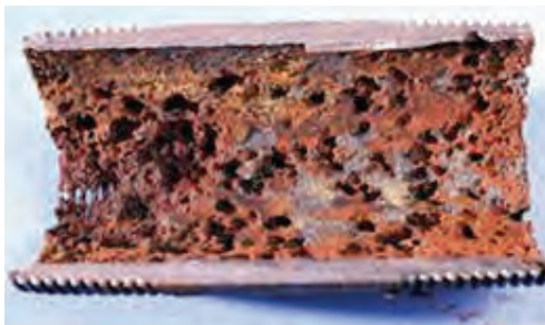
Figure 9.2.12. Condensate pipe – oxygen pitting
