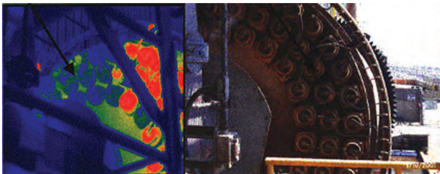
Figure 6.2.9. Inoperable steam heaters seen by cooler blue areas when compared to the operating heaters warmer red or orange colors.
