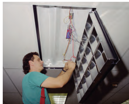
Figure 9.12.4. Repair and rewiring must be done by a licensed electrician.
