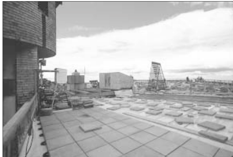
When the roof membrane was replaced on the Mount Washington Visitor Center in New Hampshire, the Styrofoam ® insulation was able to be reused because it was a protected-membrane roof.
