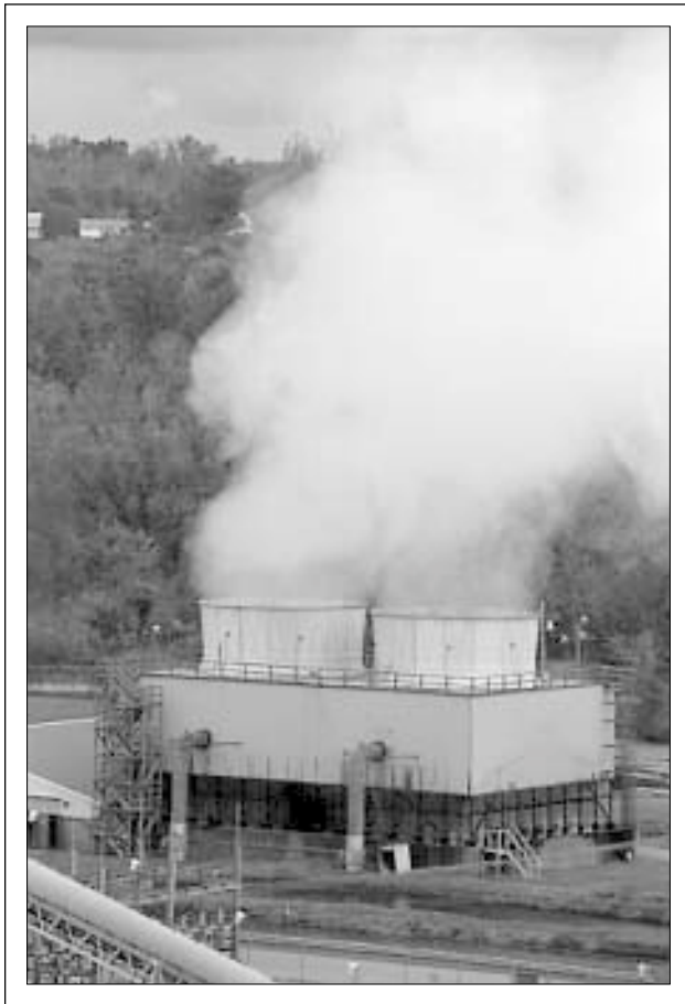
NREL worked with state, community, business, and utility partners to assist in the development of the 50-MW McNeil Generating Station in Burlington, Vermont, which uses wood fuel to produce electricity (cooling towers and excess steam are shown here).
