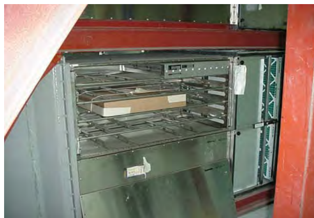
Figure G-6. Two 1,200-cfm M49 Assemblies Installed with HEPA Filters and Prefilters
