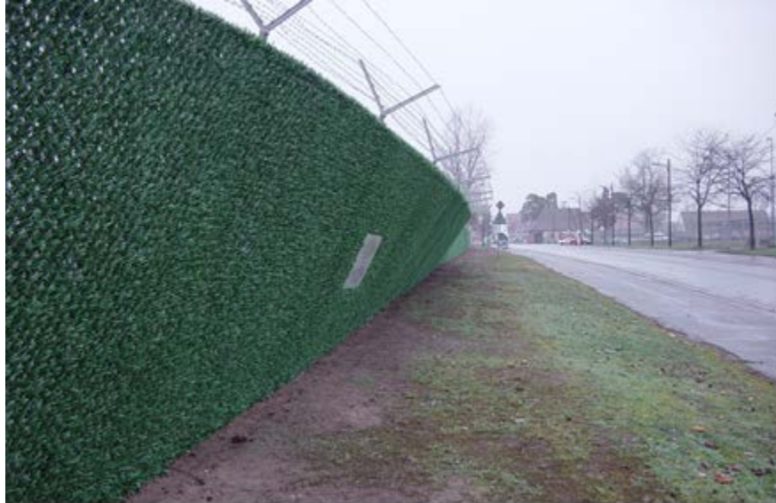
Figure 4-3. Failed Chain Link Fence with Obscuration Material Added
