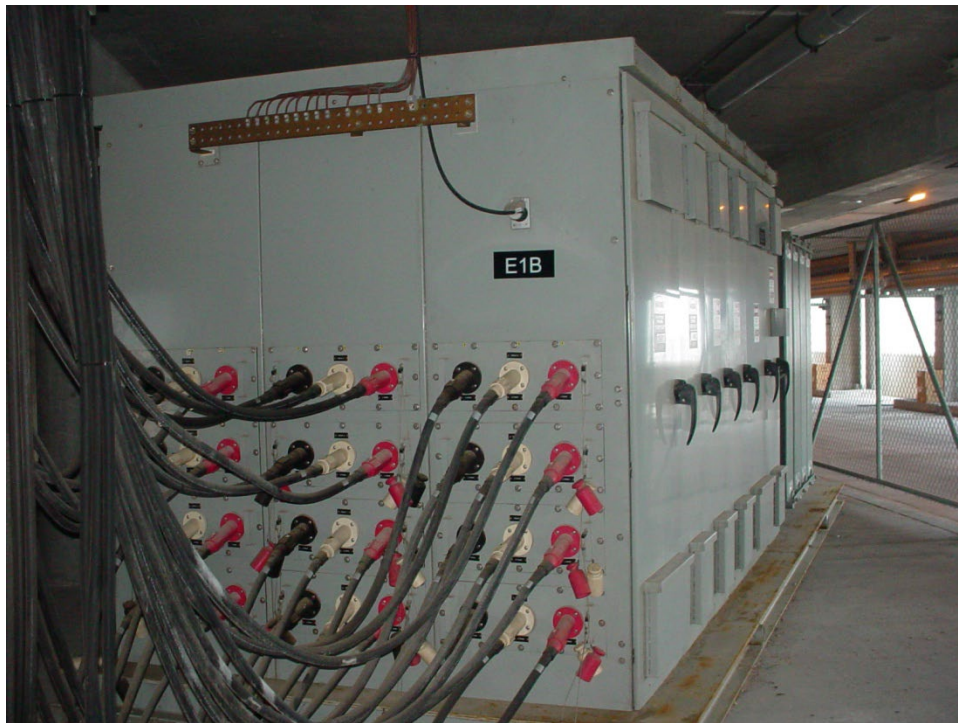
Figure 12-6. Double-Deck Pier Switchgear
