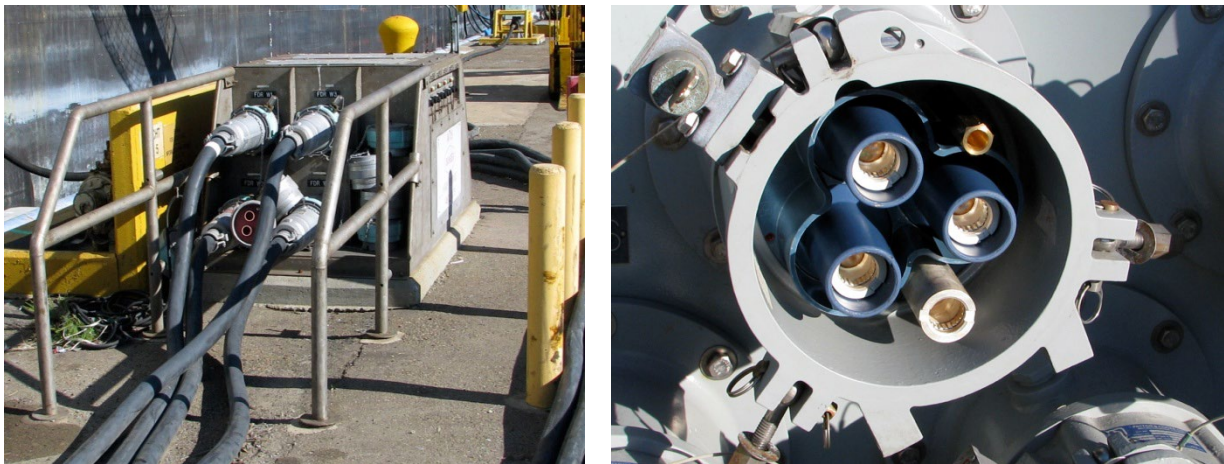
Figure 12-9. 4.16 kV Pier Electrical Outlet Assembly and Outlets – Newer Designs
