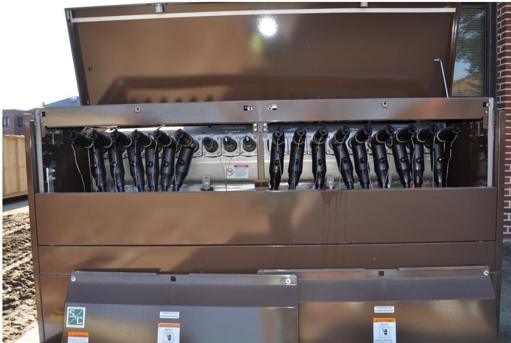
Figure D-1 S&C Vista Switchgear
