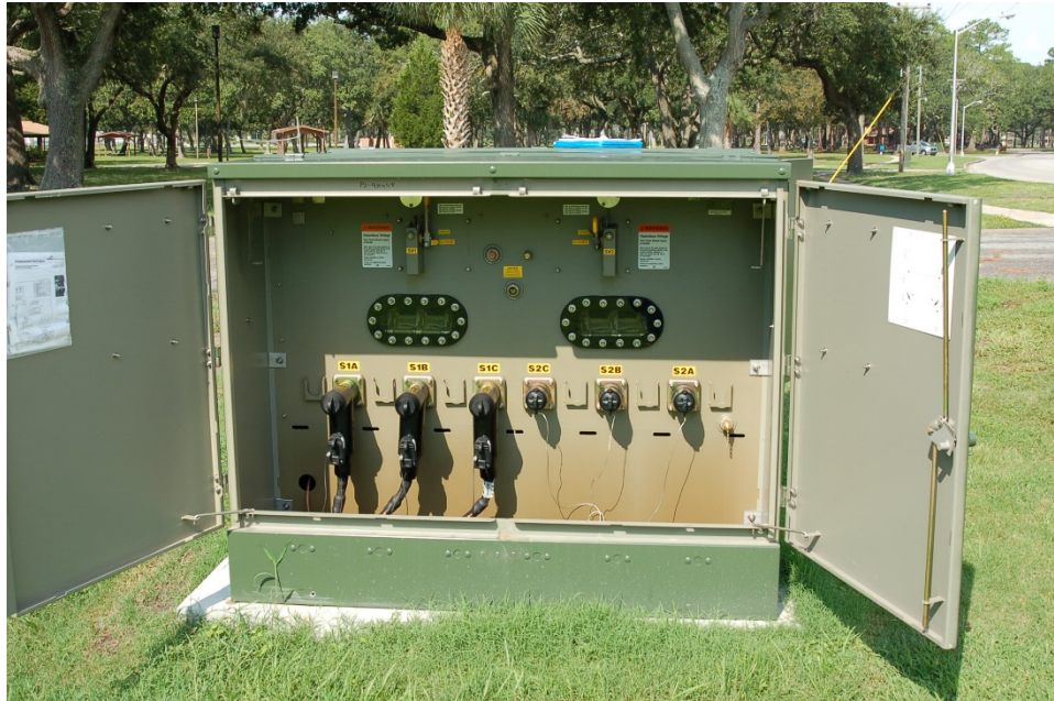
Figure D-3 Cooper VFI Switchgear
