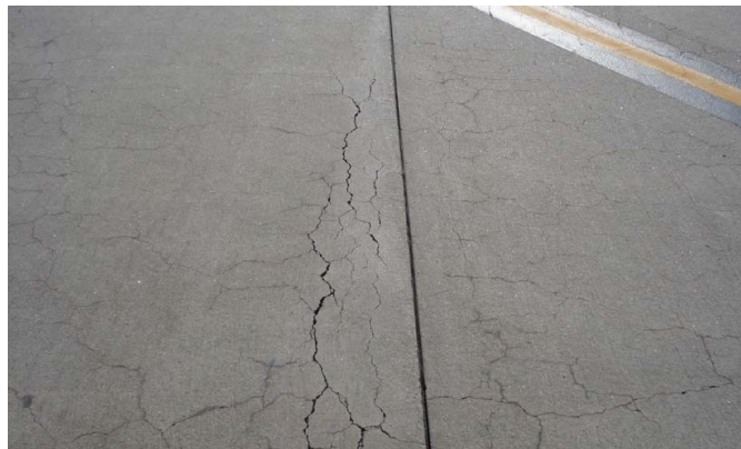
Figure 3-11 ASR Distress (Scaling/Map Cracking) on Concrete Pavement
