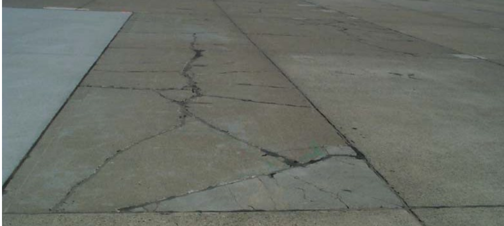
Figure 3-12 Shattered Slabs on Concrete Pavement
