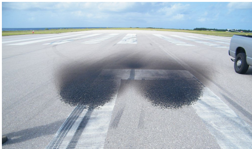
Figure 3-2 Jet Blast Damage
