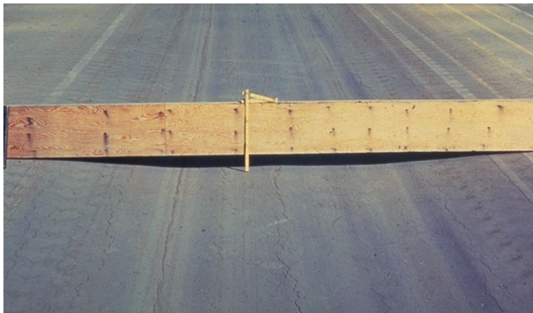
Figure 3-8 Rutting of the Pavement Structure
