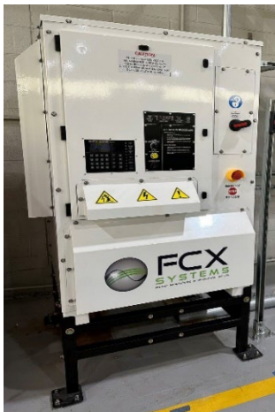
Figure 3-3 - Recent Converter Installations (270 VDC & 400 Hz) – Example 3
