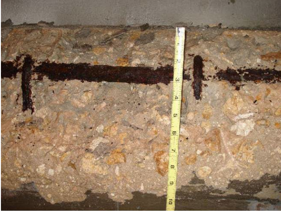
Figure 4-15. Shows a typical section of exposed corroded rebar.
