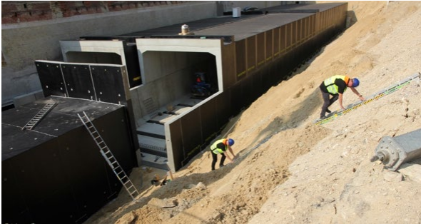
3,000 m 3 chilled-water PTES in Frederiksberg Forsyning, Carlsberg City, Denmark (Ramboll)
