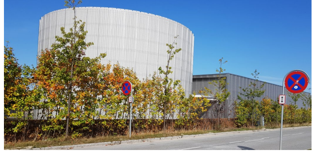
2,000 m 3 chilled-water TTES, Taarnby Forsyning, Denmark (Ramboll)
