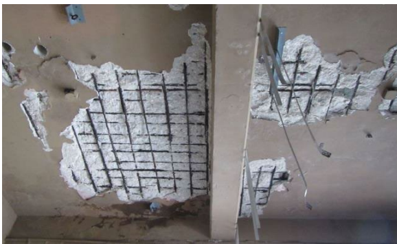
Figure 1-7. Common spalling of concrete.
