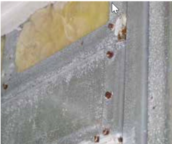
Figure 1-4. Example of corroded fasteners.
