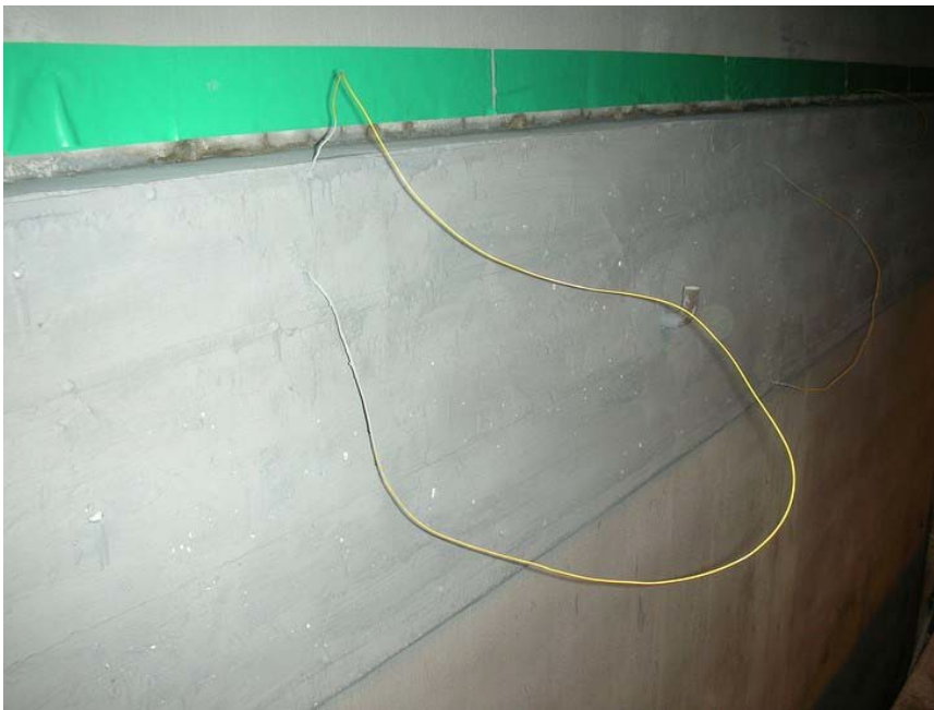
Figure B-17. The LGC application was finished when inspection showed that all concrete surfaces were uniformly covered.
