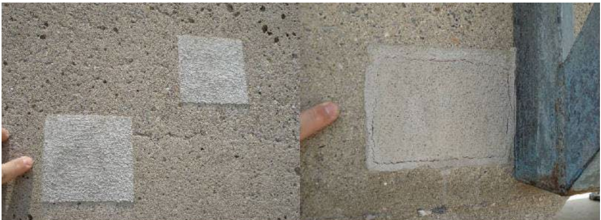
Figure 4-12. Typical repairs using a cementitious material. The patch material has a rough appearance and failed within months of installation.
