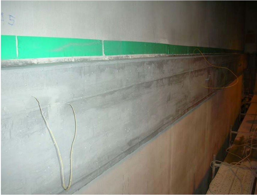
Figure B-16. Finished appearance of the Ring Girder Side 2 following application of the LGC.
