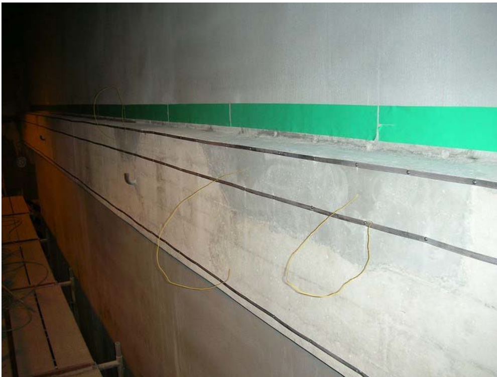
Figure B-15. Appearance of the Ring Girder Side 2 immediately after application of the LGC.
