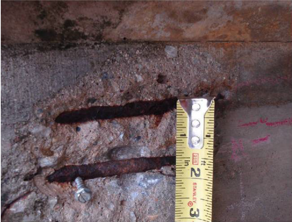
Figure 4-11. Exposed rebar on culvert.
