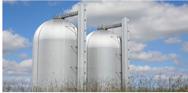
2 x 24,000 m 3 pressurized hot water TTES in Copenhagen Denmark, up to 257.0 °F (125 °C) sectioned from network by 10 Bar (Ramboll)
