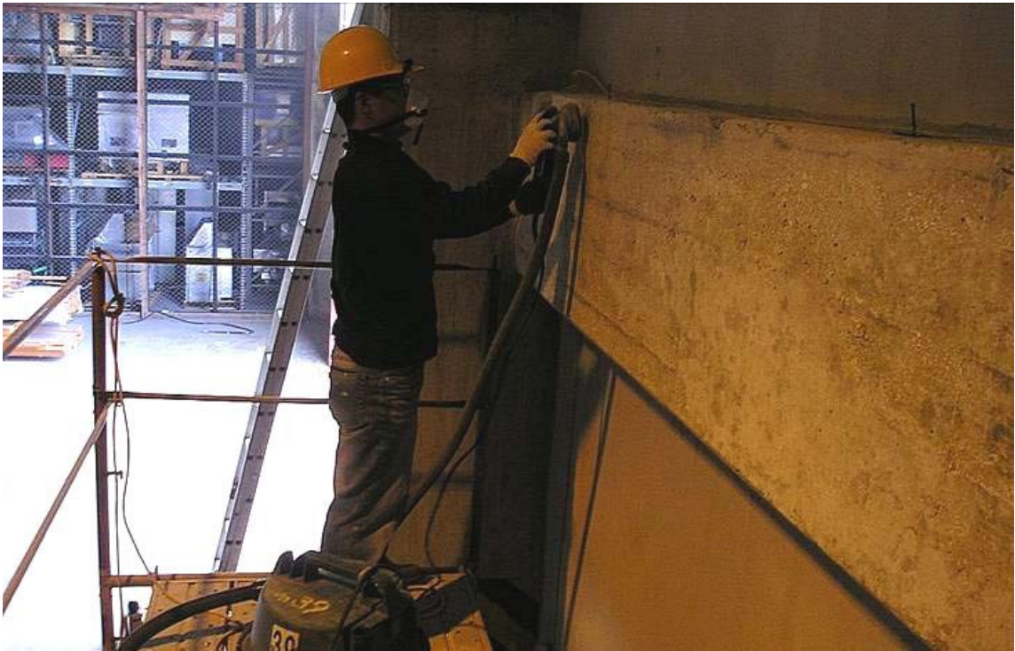
Figure B-3. Failed existing repairs; new delaminated areas were demolished.
