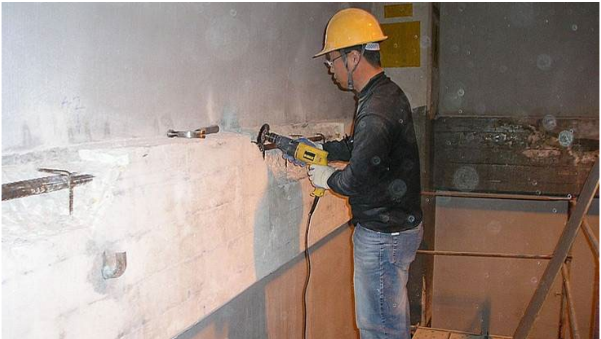
Figure B-5. Exposed rebar in repair areas cleaned by using wire wheel.
