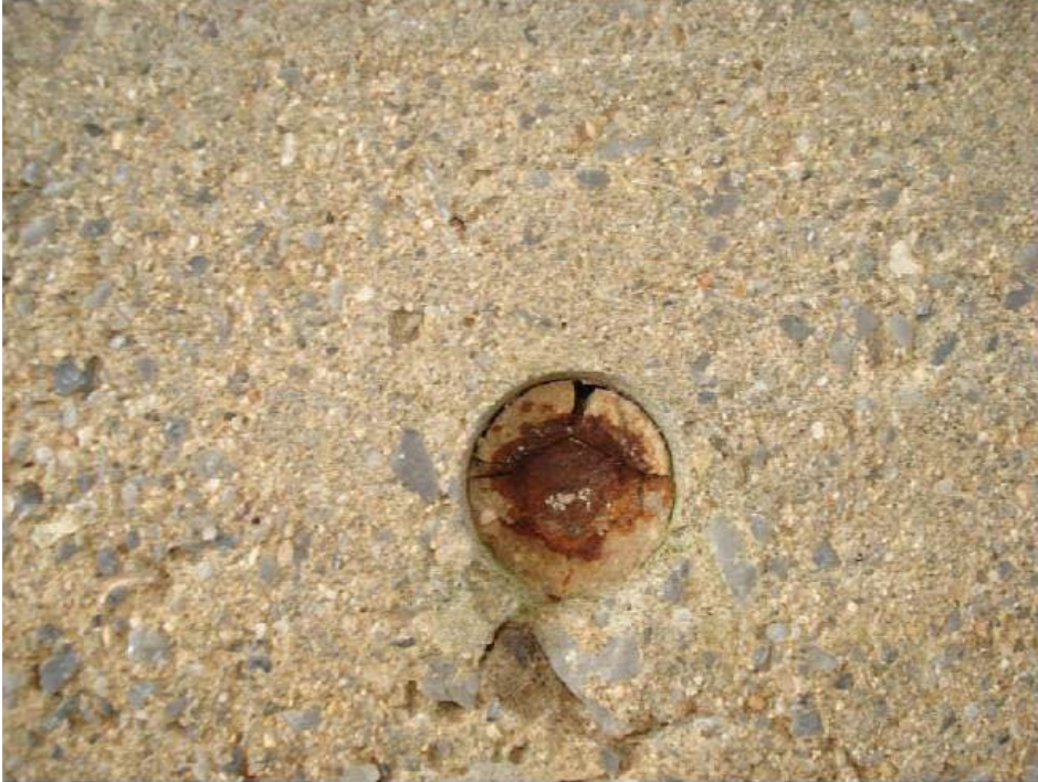
Figure 4-13. Shows a typical corroded steel rebar that has delaminated from the concrete.
