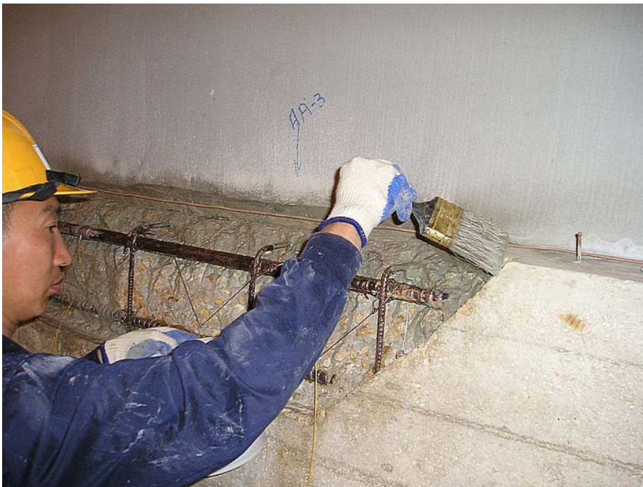
Figure B-10. Concrete repairs were placed and finished in accordance with generally accepted construction practices in all locations on the ring girder side 1 (Surtreat system).
