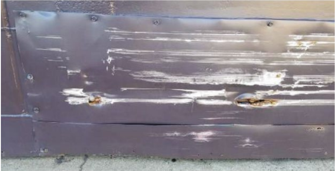
Figure 1-6. Door damage by machinery impact.
