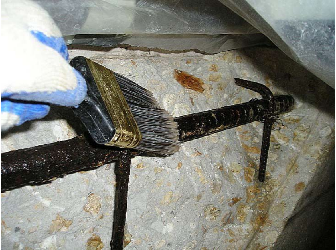
Figure B-6. Organic vapor phase corrosion inhibitor applied to all demolished delamination areas.
