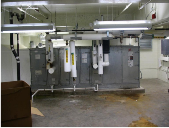
Figure 1-14. Mechanical room at Fort Bragg.
