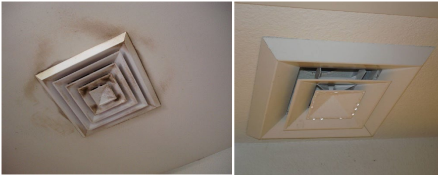
Figure 5-18. Condensation on ceilings and diffusers.
