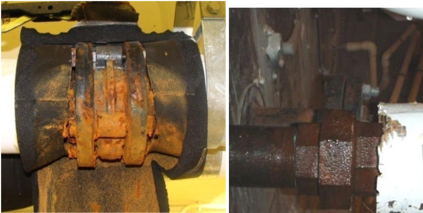
Figure 1-15. Corroded union joints on piping in a mechanical room.
