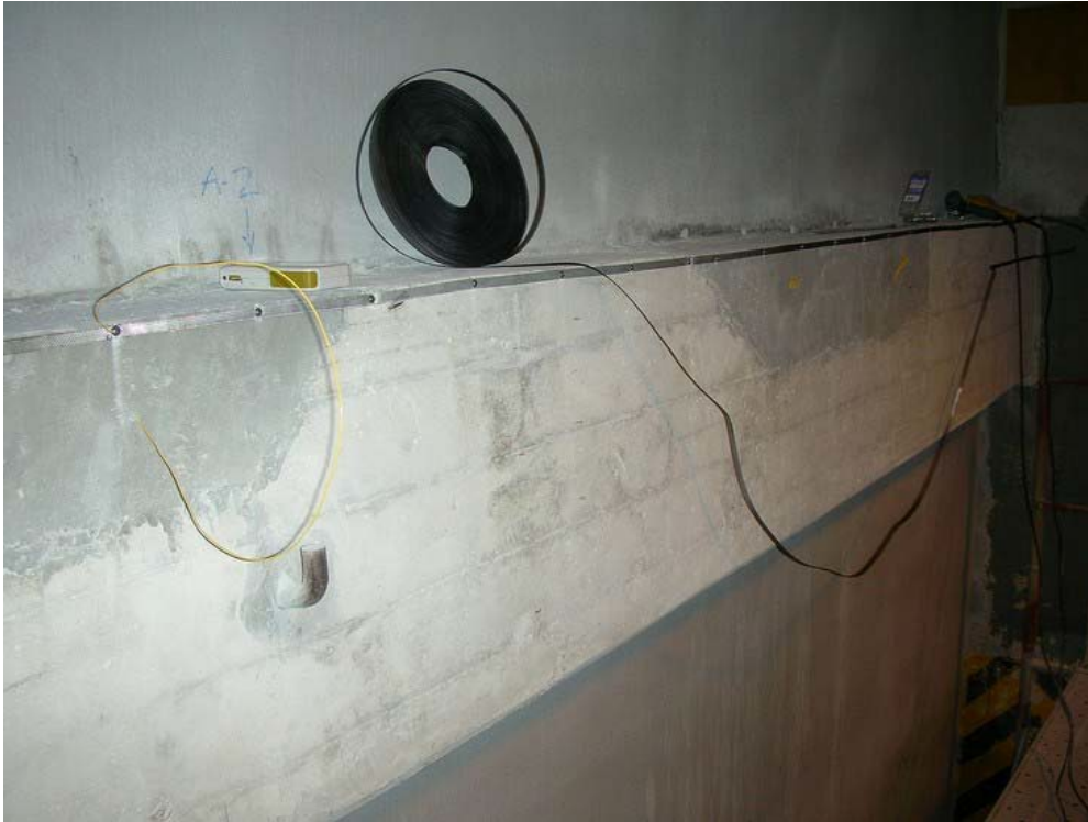
Figure B-14. Appearance of the Ring Girder Side 2 before application of the LGC.
