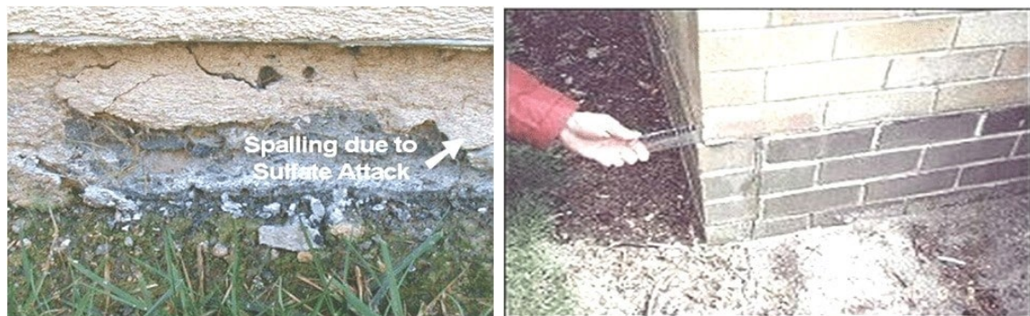
Figure 1-12. Spalling due to a sulfate attack.
