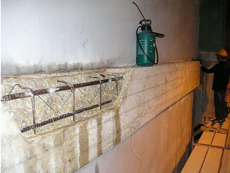
Figure B-7. Electrical connections to the rebar were made to facilitate future testing.
