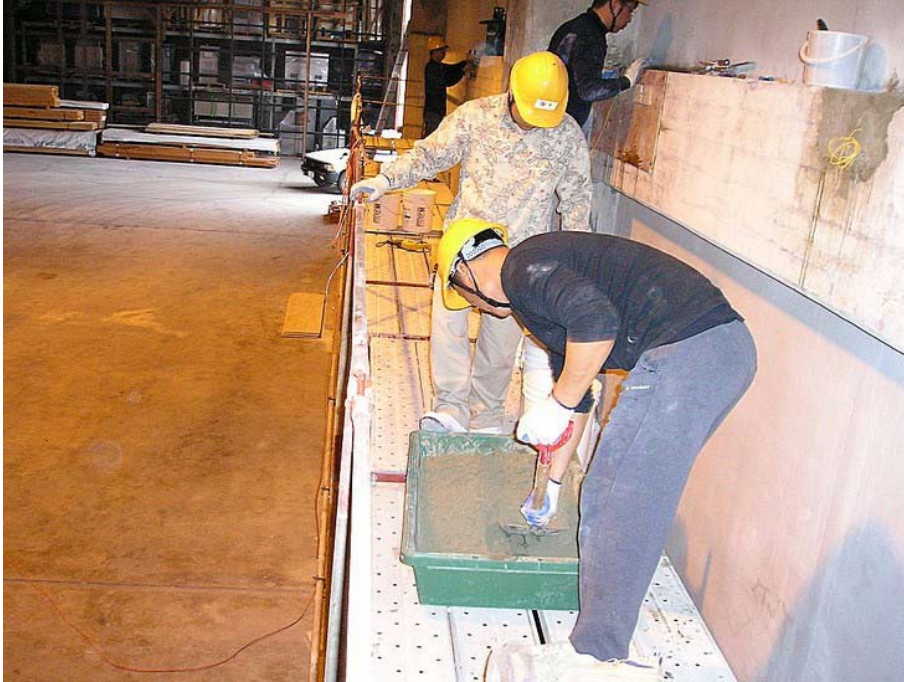
Figure B-9. Concrete repairs were made following corrosion inhibitor system application to the demolished delamination areas.
