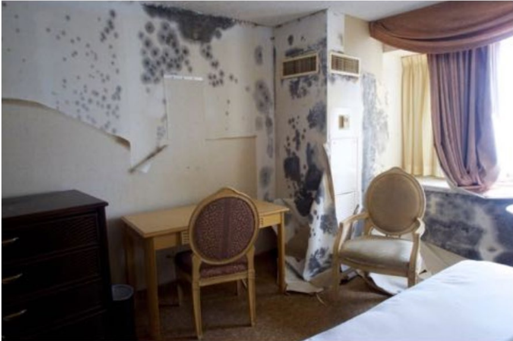
Figure 4-5. Moisture trapped by an interior vinyl wallpaper vapor barrier.
