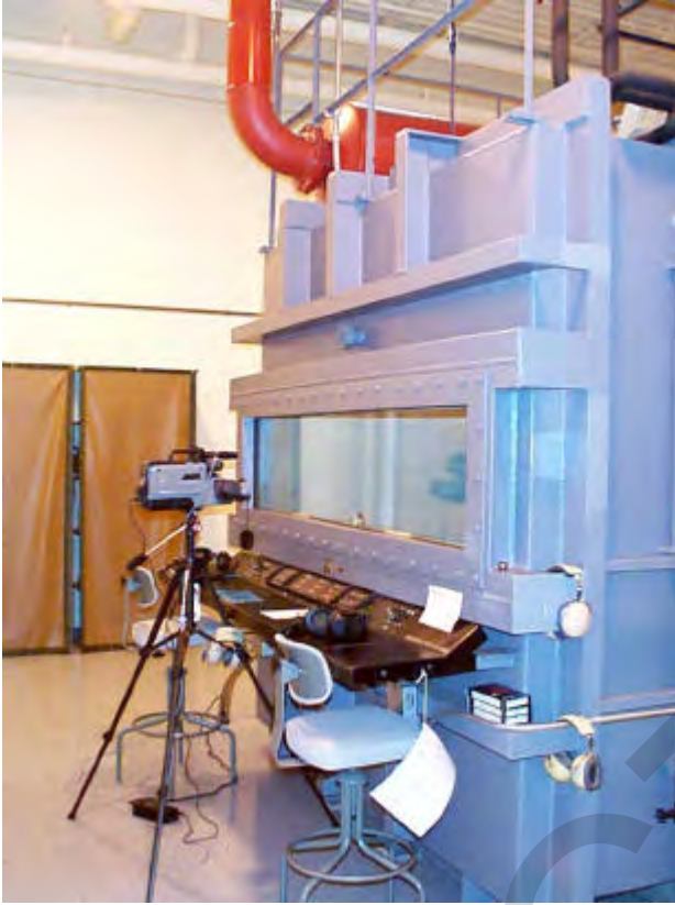
PHOTO 4 Decompression Chamber - Front Elevation
