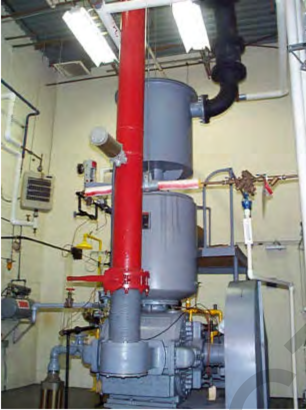
PHOTO 6 Vacuum for Decompression Chamber
