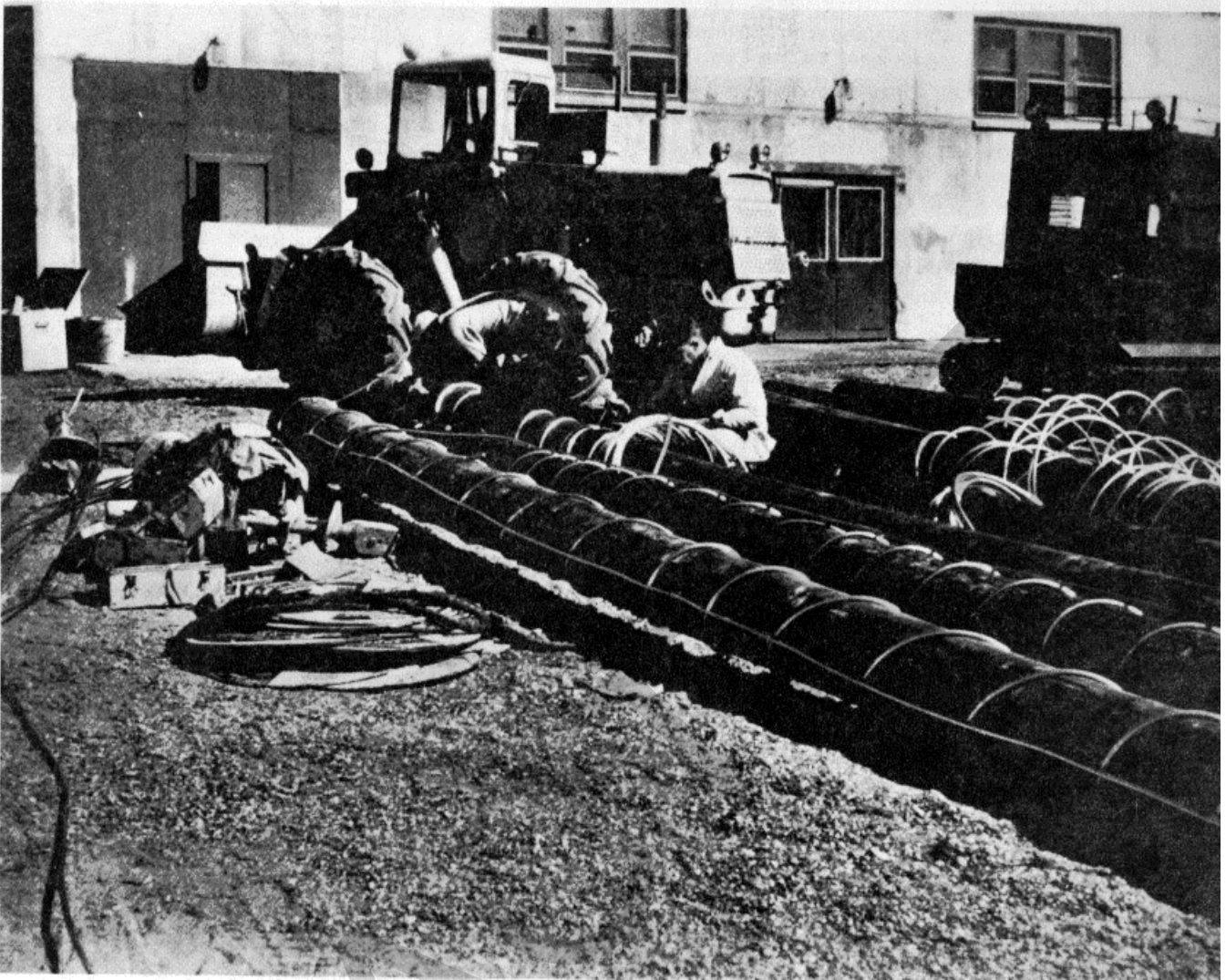
Figure 4-75. Refrigeration coils on timber piles for artificial freezeback.
