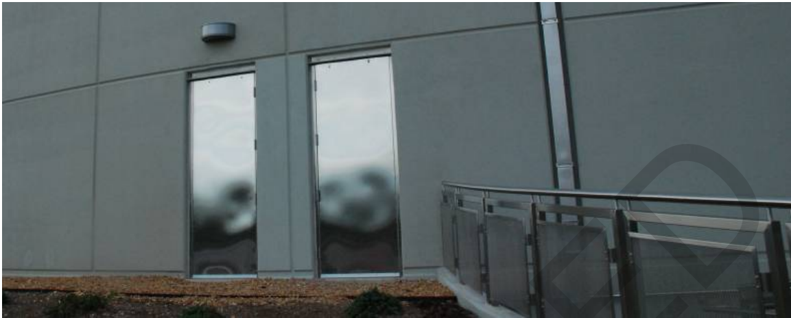
Figure 3-5 Emergency Exit Doors
