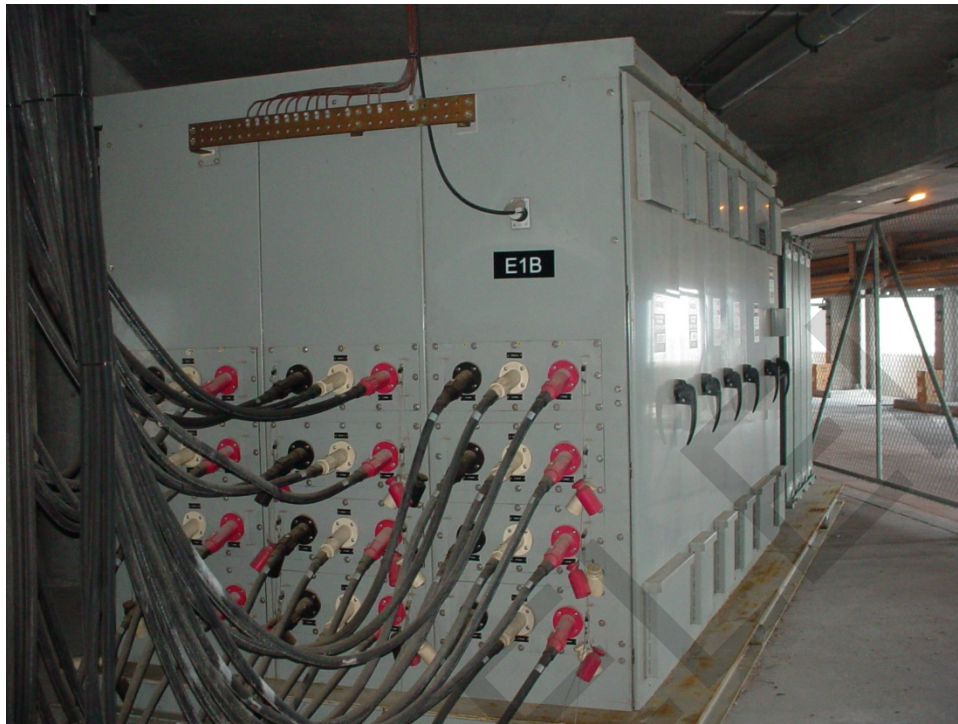
Figure 12-6. Double-Deck Pier Switchgear
