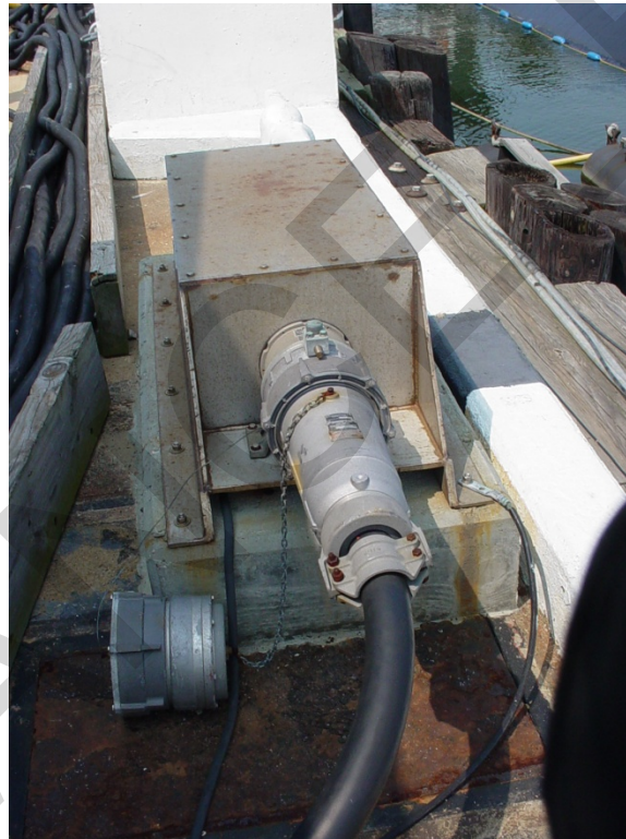
Figure 12-1. Electrical Connection Outlet Assembly with a 15 kV Receptacle
