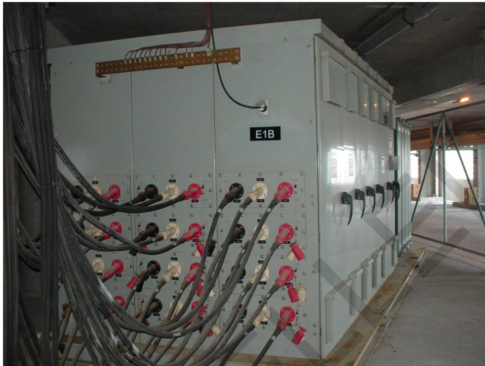
Figure 12-6. Double-Deck Pier Switchgear
