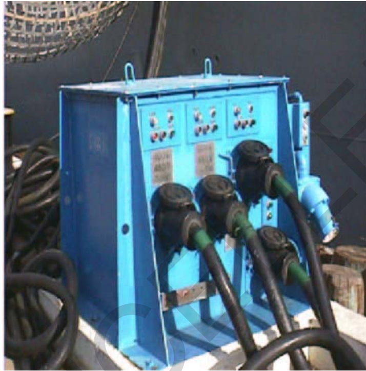
Figure 13-9. 480 Volt Pier Electrical Outlet Assembly and Cable Connections
