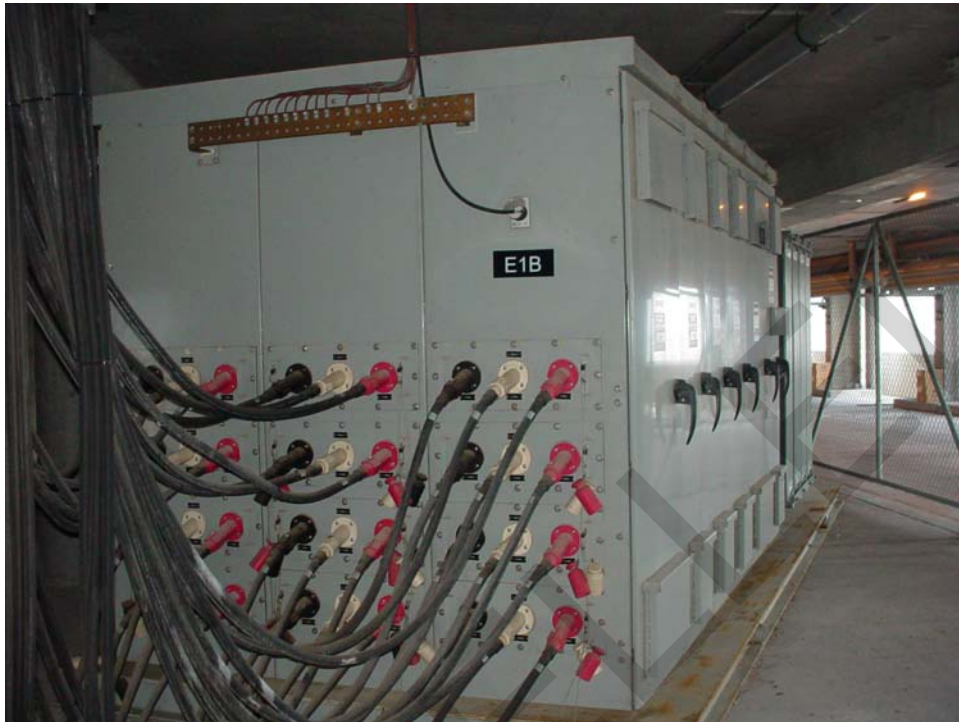
Figure 13-6. Newer Double-Deck Pier Switchgear
