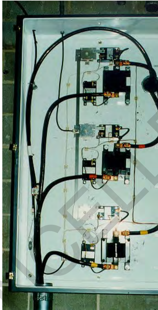
Figure D-4. Excessive Lead Length Caused by Over-Sized Enclosure
