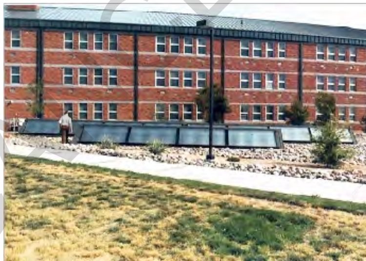
Figure G-1. Photo of Collector Arrays
