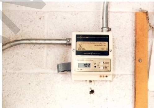
Figure G-8. Differential Temperature Controller
