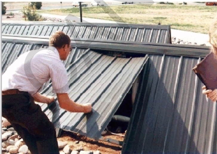
Figure G-6. Equipment Housing
