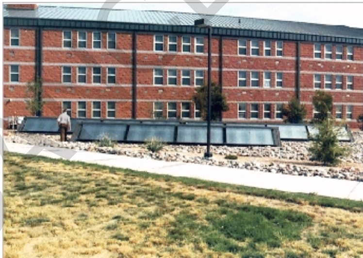
Figure G-1. Photo of Collector Arrays
