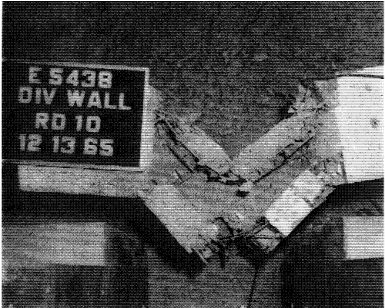
Figure 4-70 Failure at Plastic Hinges of Laced Elements
