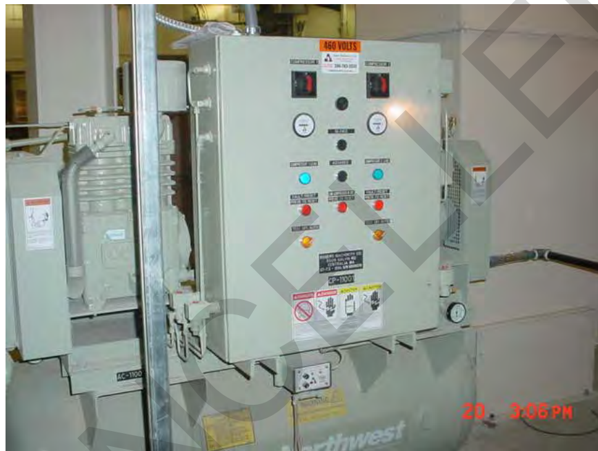
Figure 3-5. Control Panel Mounted on Top the 120-Gallon Air Tank
