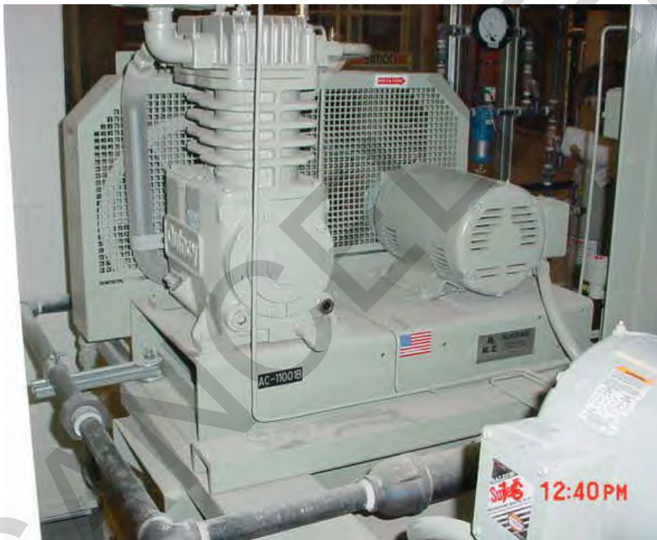
Figure 3-4. One of Two Motor Driven Reciprocating Compressors
