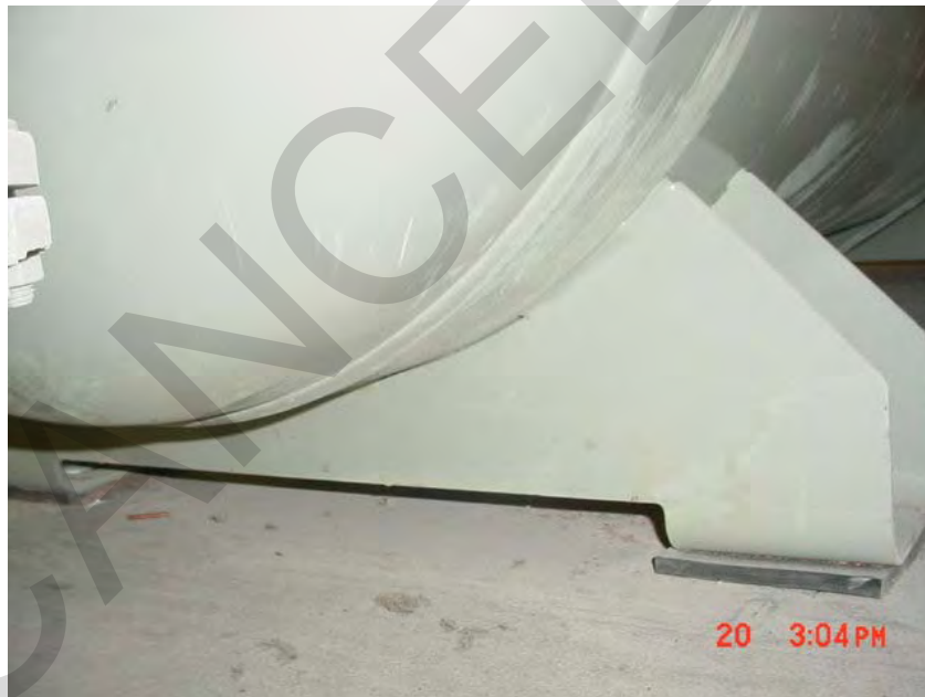
Figure 3-6. 120 Gallon Air Tank Sit on Neoprene Isolator Pads
