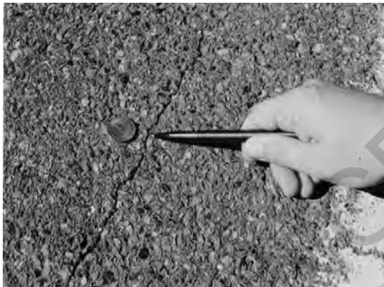
Figure 7.1. Example of hairline-size crack
