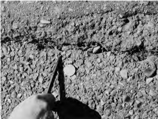
Figure 7.3. Example of a medium-size crack
