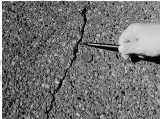
Figure 7.2. Example of a small-size crack
