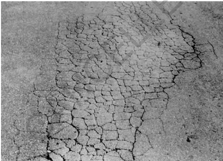
Figure 2.1. Example of alligator cracking
