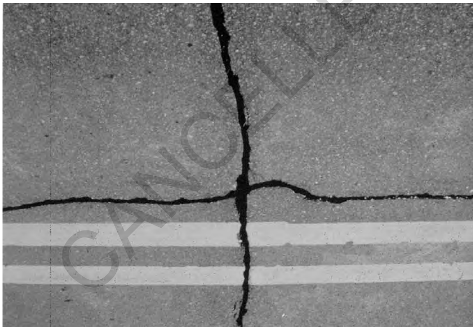
Figure 9.5. A crack after sealing
