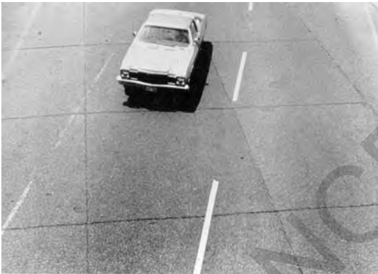
Figure 3.1. Example of reflective cracking
