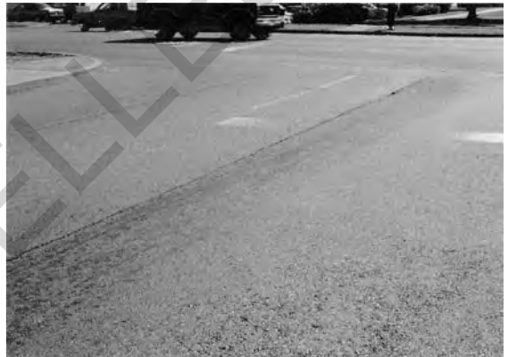
Figure 3.2. Example of longitudinal cracking
