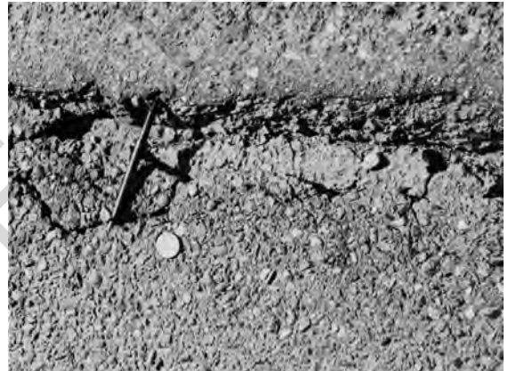
Figure 7.4. Example of large-size crack
