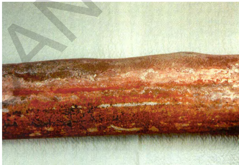
Figure 3-7. Metal Fatigue on Boiler Tube
