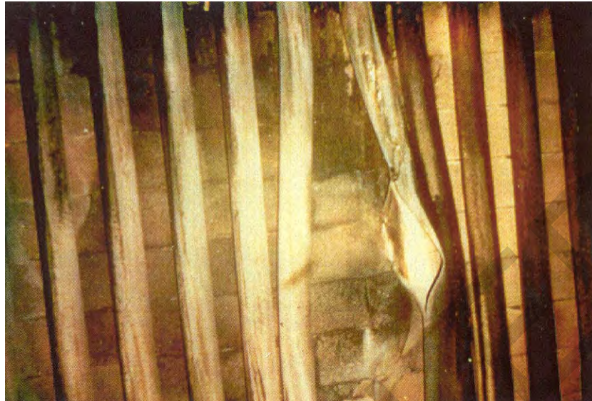
Figure 3-8. Failed Boiler Tube
