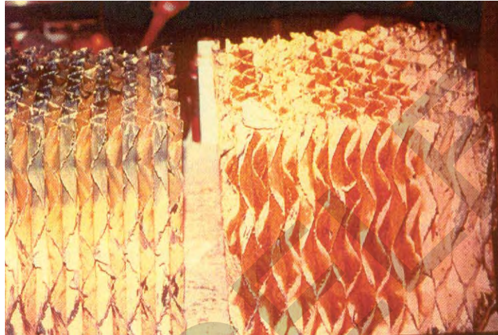
Figure 4-14. Heavily Fouled Cooling Tower Film Fill
