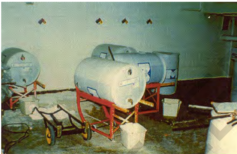
Figure 7-2. Manual Chemical Feed System
