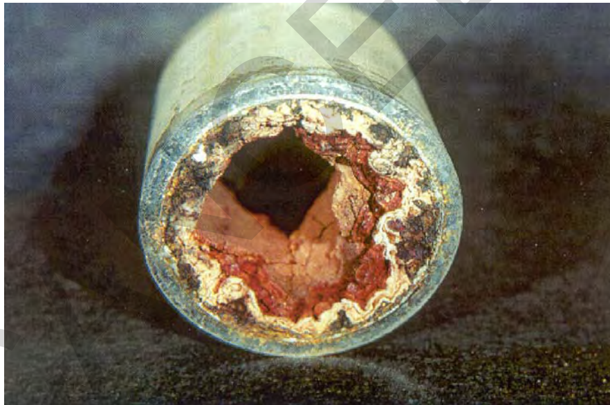
FIGURE 3-5. Scaled Boiler Tube
