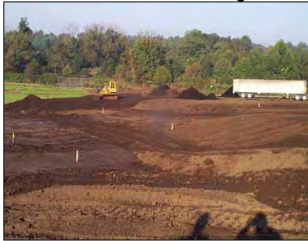
Figure 8-1. Southern Maryland Wood Treating Site: On-site Thermal Desorption of Contaminated Soils. Final Grading and LeafGro® Placement
