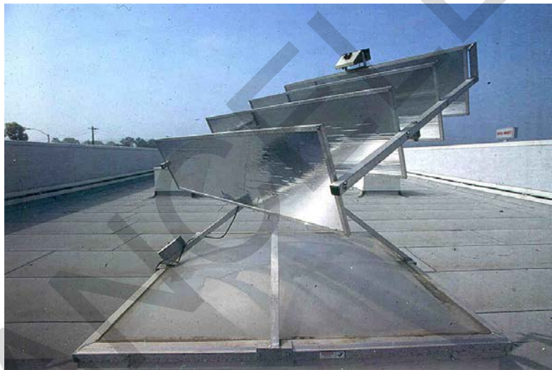
Figure C-11 Example of an Active Daylighting System that Tracks the Sun and Directs Daylight into the Building.
