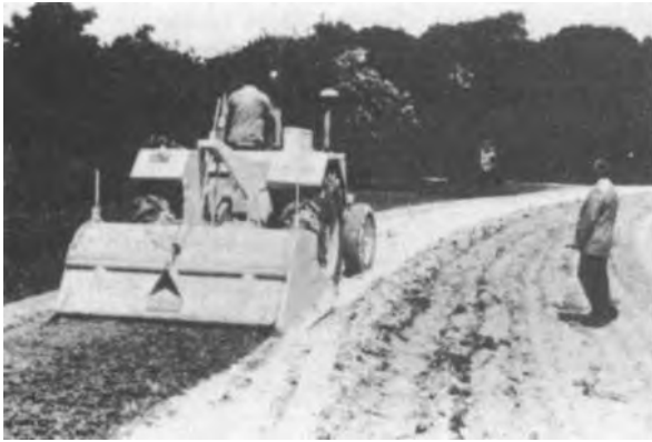
Figure 4-15. In-place mixing of lime with existing base and paving material on city street.
