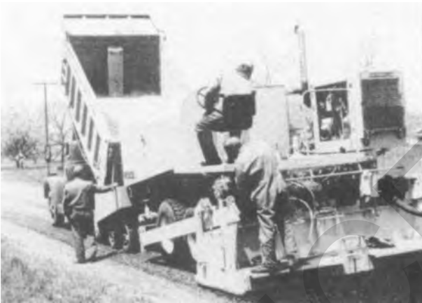
Figure 4-45. Hopper-type pugmill travel plant.
