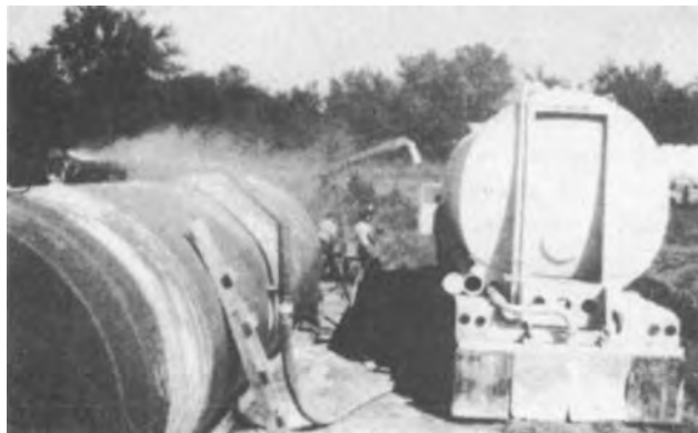
Figure 4-29. Slurry mixing tank using recirculating pump for mixing hydrate and water.
