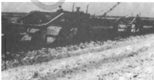
Figure 4-38. Train of rotary mixers.
