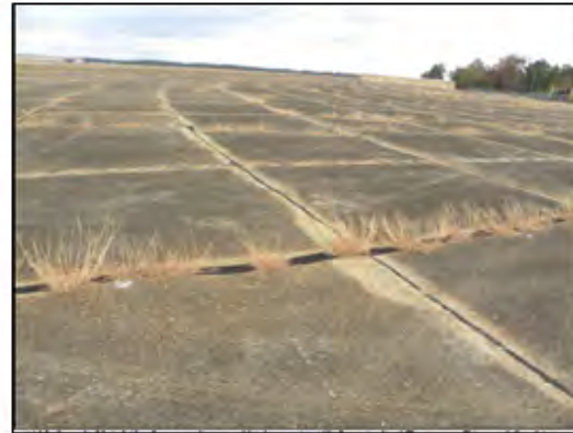
Photo 8, Typical Joint Seal Damage and Joint Spalling on Section A01B
