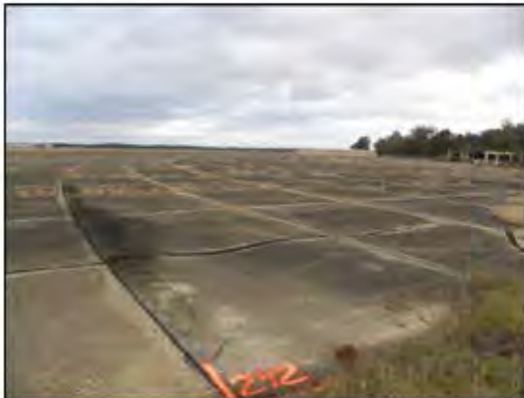
Photo 9, Longitudinal/Transverse Cracking and Joint Spalling on Section A01B
