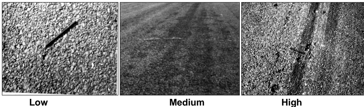
Figure B-15 Raveling, Porous Friction Course Severity Levels
