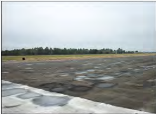
Photo 3, Low Severity Block Cracking on Section R04A, RWY 08/26
