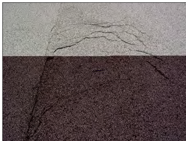
Figure B-1 Slippage Cracking
