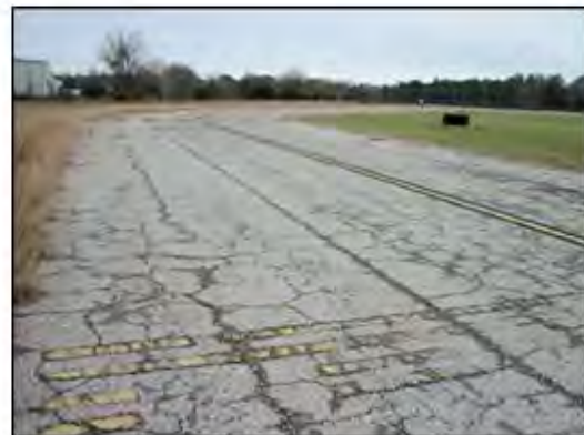
Photo 6, Medium Severity Block Cracking and Raveling on Section T07A
