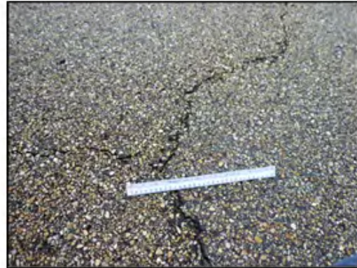
Photo 2, Typical Medium Severity Transverse Cracking and Low Severity Weathering on Section R02C, RWY 18/36
