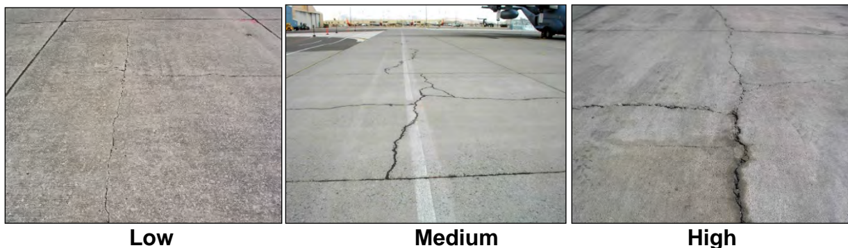
Figure C-13 Shattered Slab/Intersecting Cracks Severity Levels
