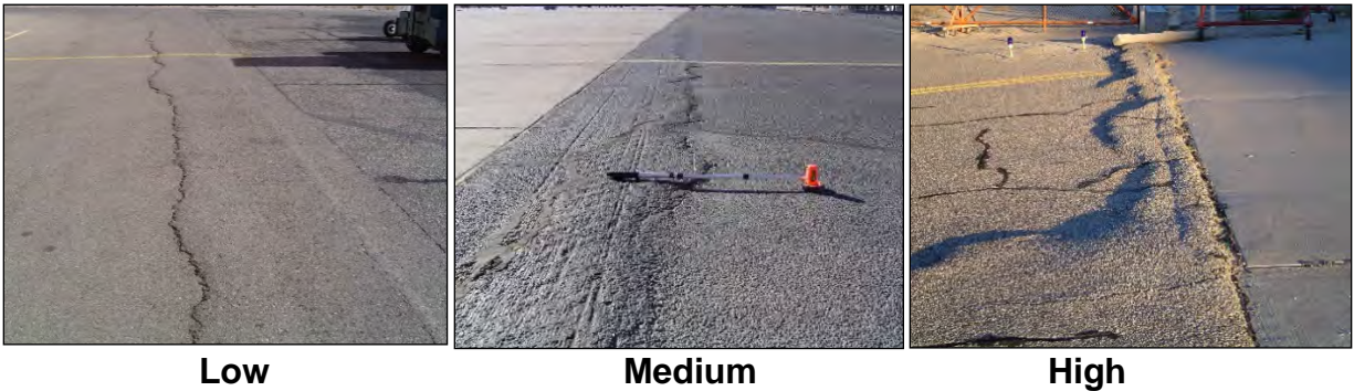
Figure B-17 Shoving Severity Levels
