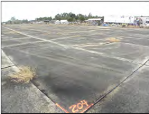
Photo 7, Longitudinal/Transverse Cracking, Joint Seal Damage, and Joint Spalling on Section A01B
