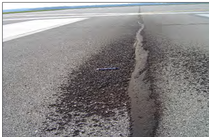
Figure B-6 Jet Blast Erosion
