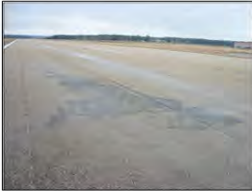
Photo 1, Typical Low Severity Longitudinal Cracking on Section R02C, RWY 18/36
