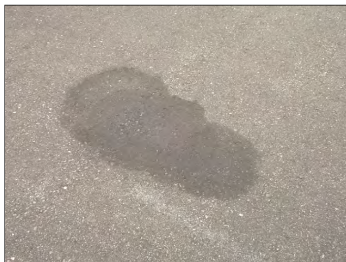
Figure B-10 Oil Spillage
