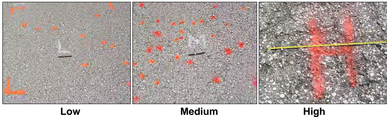
Figure B-13 Raveling, Dense Mix Severity Levels
