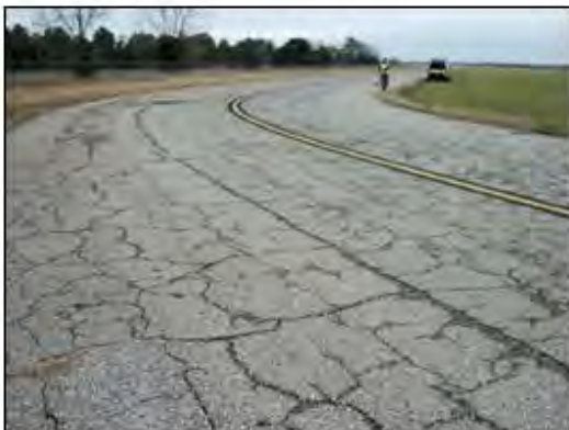
Photo 5, Medium Severity Block Cracking and Raveling on Section T07A
