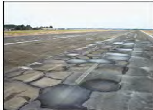
Photo 4, Medium Severity Block Cracking on Section R05C, RWY 08/26 (Note the Curling Edges)
