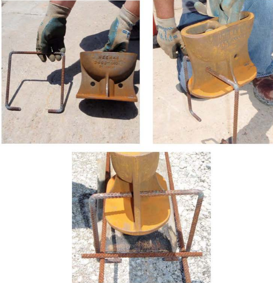
Figure 9. Neenah With Bent Rebar for Installation in HMA Pavement With Minimum 12-Inch (305-mm) -Thick PCC Underlay.
