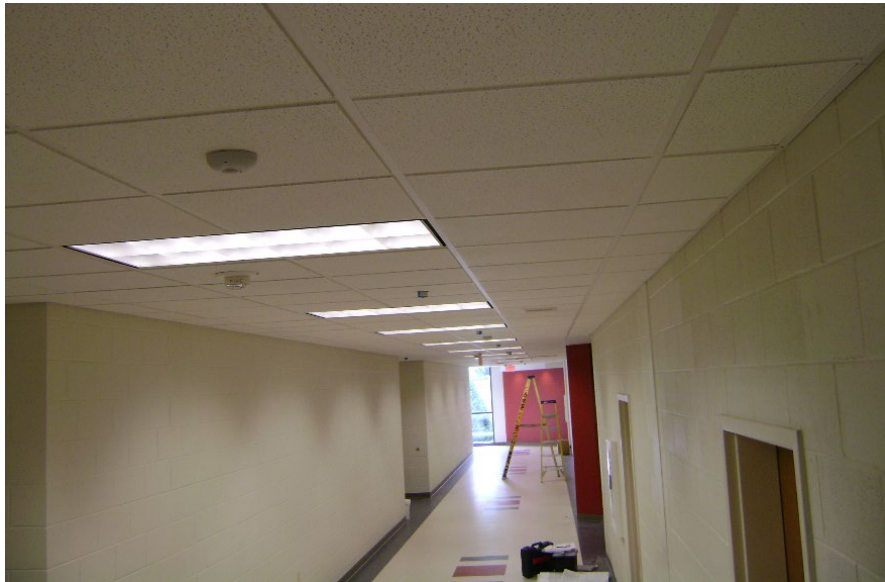
Figure 4-12 Finished Center of Tile Installation Using Flexible Sprinkler Hose Fittings (Courtesy of TERPconsulting)
