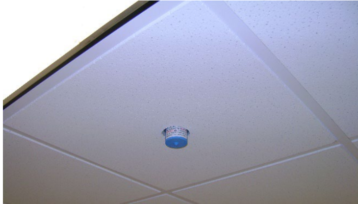
Figure 4-3 Center-of-Tile Installation Using Flexible Sprinkler Hose Fittings (Courtesy of TERPconsulting)
