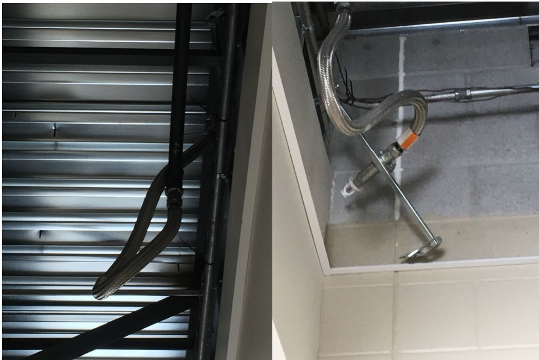
Figure 5-5 Unprotected Sprinklers Installed on Flexible Sprinkler Hose Assemblies (Courtesy of TERPconsulting)
