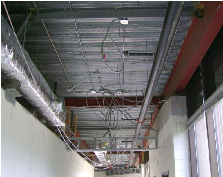
Figure 4-5 Rough-In Installation for Flexible Sprinkler Hose Fittings (Courtesy of TERPconsulting)
