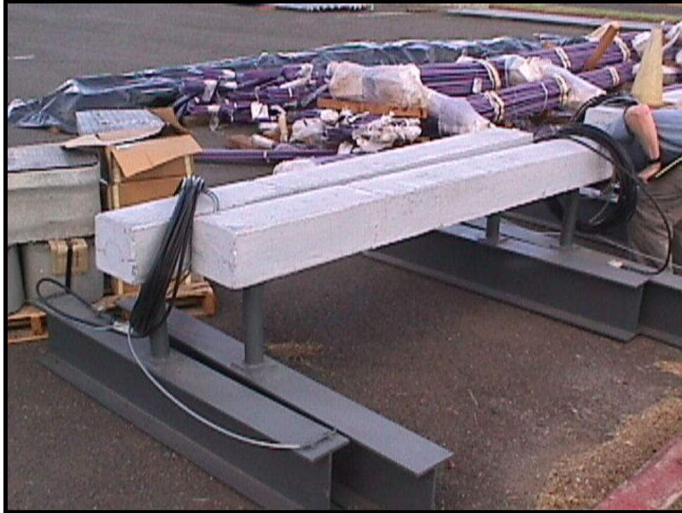
Figure 8 Large aluminum anodes for sheet pile bulkhead
