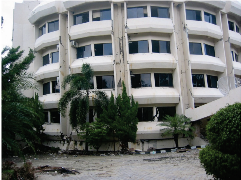
(b) Soft story failure
