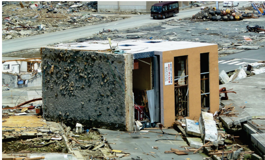
Figure 2-30 Overturned three-story commercial building on a mat foundation in Onagawa, Japan, 2011 Tohoku tsunami (photo courtesy of I. Robertson and ASCE, from Chock, et al., 2013b).
