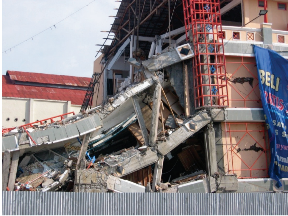
(a) Beam-column connection failures
