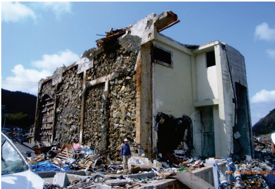
Figure 2-28 Overturned cold storage building in Onagawa, Japan, 2011 Tohoku tsunami (photo courtesy of G. Chock and ASCE, from Chock, et al., 2013b).
