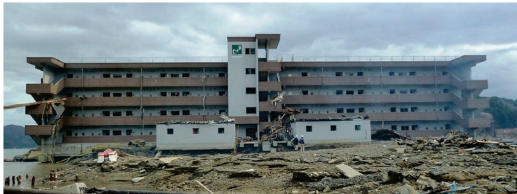
Figure 6-2 Reinforced concrete apartment building designated as a vertical evacuation structure in Minamisanriku, Japan, 2011 Tohoku tsunami.
