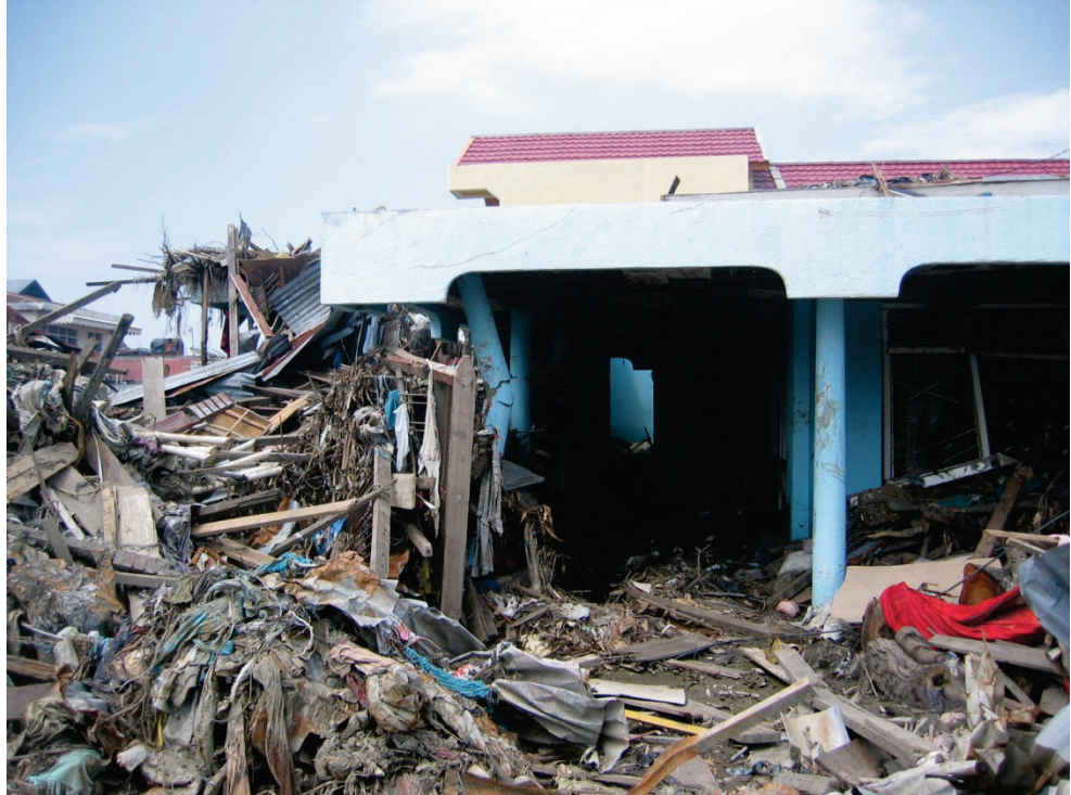
Figure 2-18 Damage to corner column due to debris damming, 2004 Indian Ocean tsunami (photo courtesy of M. Saatcioglu, A. Ghobarah and I. Nistor, CAEE, 2005).
