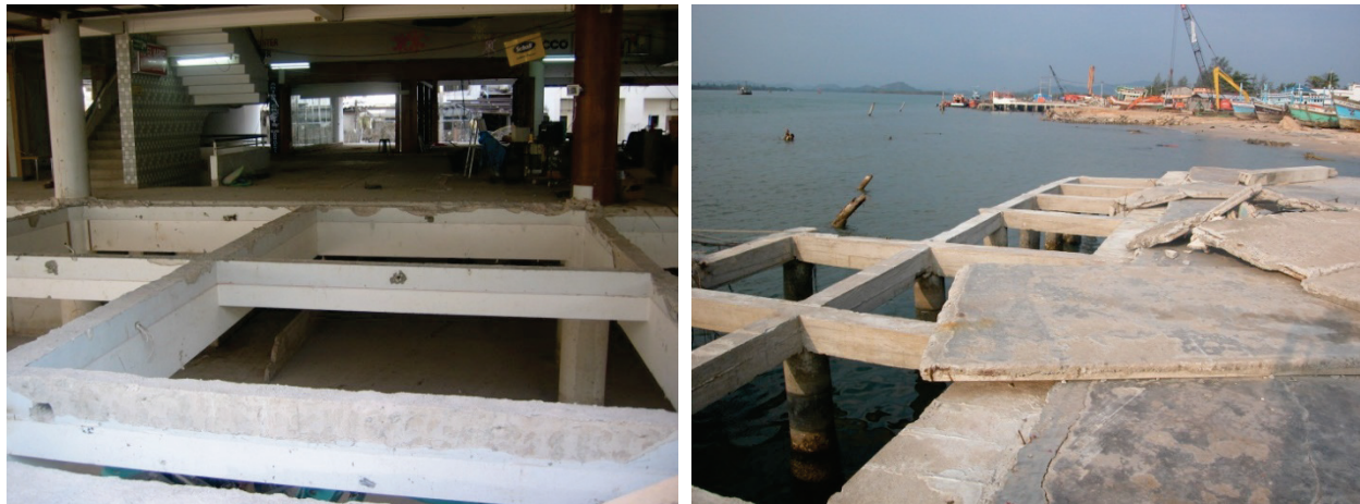
Figure 2-20 Uplift damage to precast concrete floor panels and harbor piers, 2004 Indian Ocean tsunami (photos courtesy of M. Saatcioglu, A. Ghobarah, and I. Nistor, CAEE, 2005).
