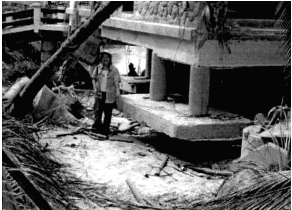
Figure 2-19 Scour around shallow spread footing in Khao Lak area, Thailand, 2004 Indian Ocean tsunami (Dalrymple and Kriebel, 2005).
