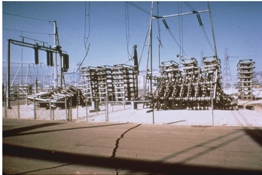
Figure 2-13 Sylmar high voltage direct current converter station damaged in the 1971 San Fernando earthquake (NOAA/NGDC, E.V. Leyendecker, U.S. Geological Survey).
