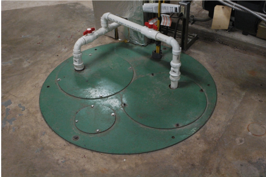
Figure 4-7 Sump cover; pump is within the sump.
