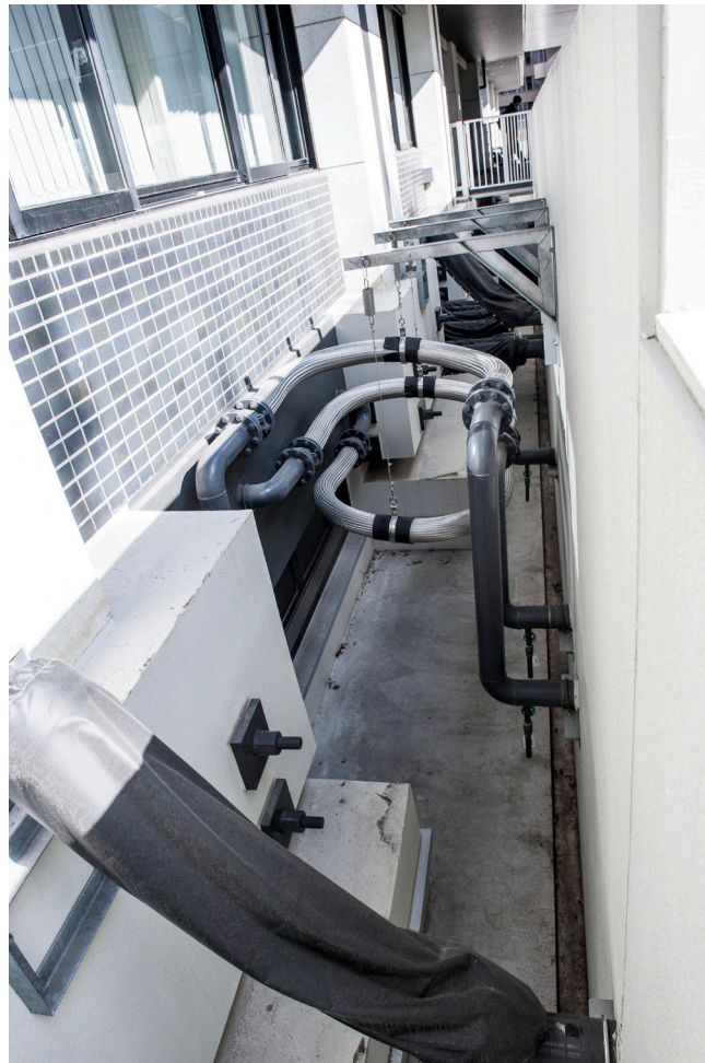
Figure 2-18 Typical flexible utility connections in base isolated building.
