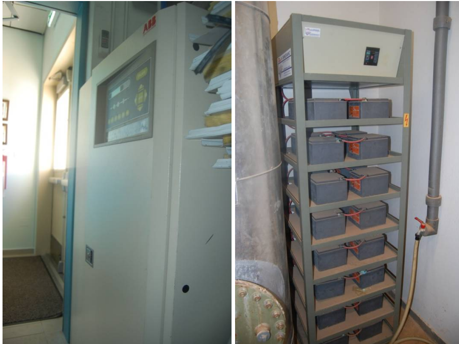
Figure 5-1 UPS system containing an inverter (left) and battery rack (right) located in a low seismic area.
