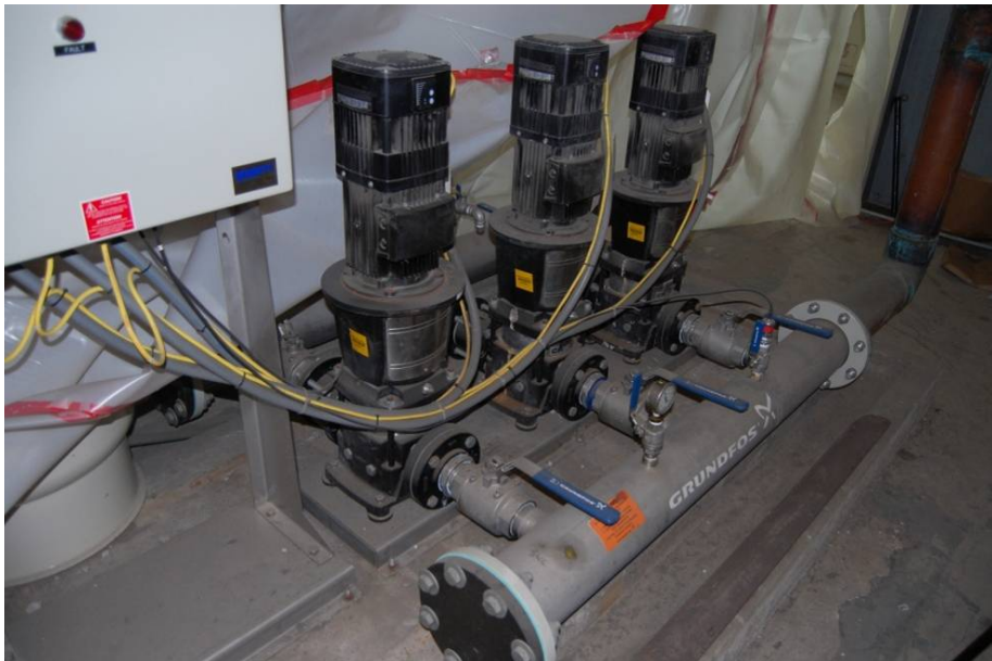
Figure 4-8 Domestic water booster pumps.
