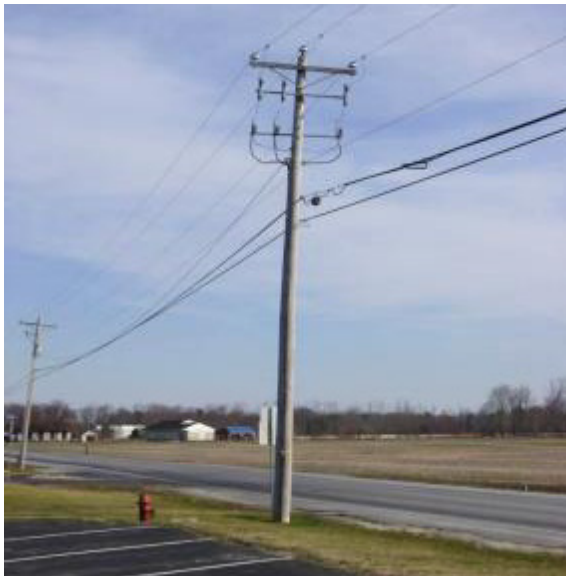
Figure 2-4 Riser pole of an underground electrical line supplied from an overhead line.
