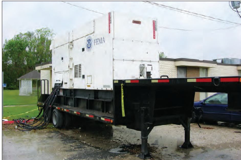
Figure 6-118: In lieu of permanent on-site emergency generators, portable generators can be an economical way to provide electrical power to schools used as hurricane recovery centers. Estimated wind speed: 108 mph. Hurricane Ike (Texas, 2008)
