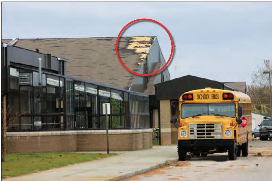
Figure 6-12: Constructed in 1995, this school was used as a hurricane shelter. The large number of occupants moved from one area of the school to another as water entered various areas of the building due to envelope failures. Estimated wind speed: 105 to 115 mph. Hurricane Ivan (Florida, 2004)
