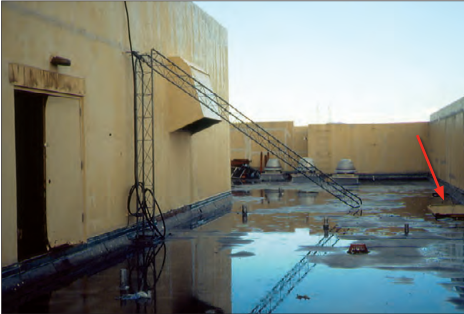
Figure 6-139: The antenna collapsed and was whipped back and forth across the roof membrane. Hurricane Andrew (Florida, 1992)
