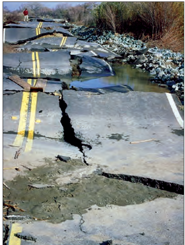
Figure 5-12: Flooding caused the failure of this road bed
