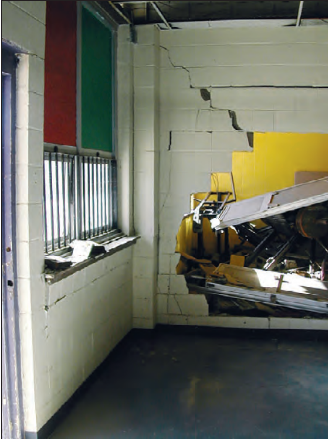
Figure 5-14: Interior unreinforced masonry walls of the Port Sulphur High School in Louisiana were damaged by hydrostatic loads associated with Hurricane Katrina's storm surge (2005)
