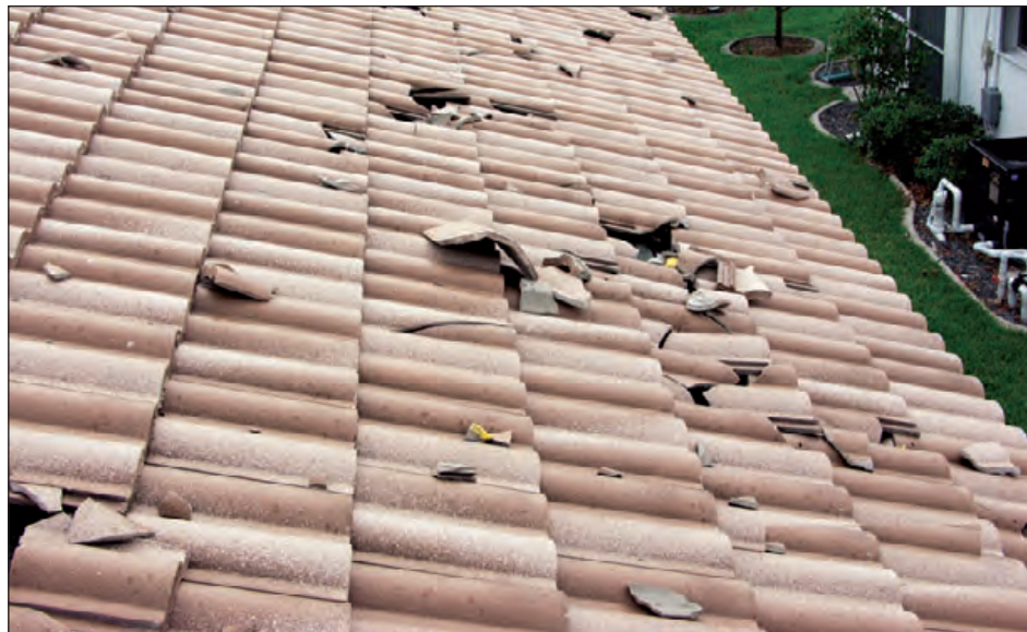
Figure 6-83: Brittle roof coverings, like slate and tile, can be broken by missiles, and tile debris can break other tiles. Estimated wind speed: 140–160 mph. Hurricane Charley (Florida, 2004)
