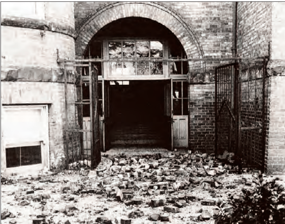
Figure 4-20: Another dangerous entry collapse, Seattle, WA, 1949
