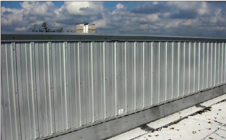
Figure 6-88: Base flashing protected by metal wall panels attached with exposed screws. Estimated wind speed: 120 mph. Hurricane Katrina (Mississippi, 2005)
