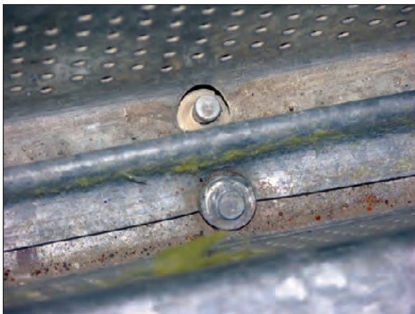
Figure 6-37: Looking down at a sidelap of a deck attached with powder-driven pins. The washer at the top pin blew through the deck.
