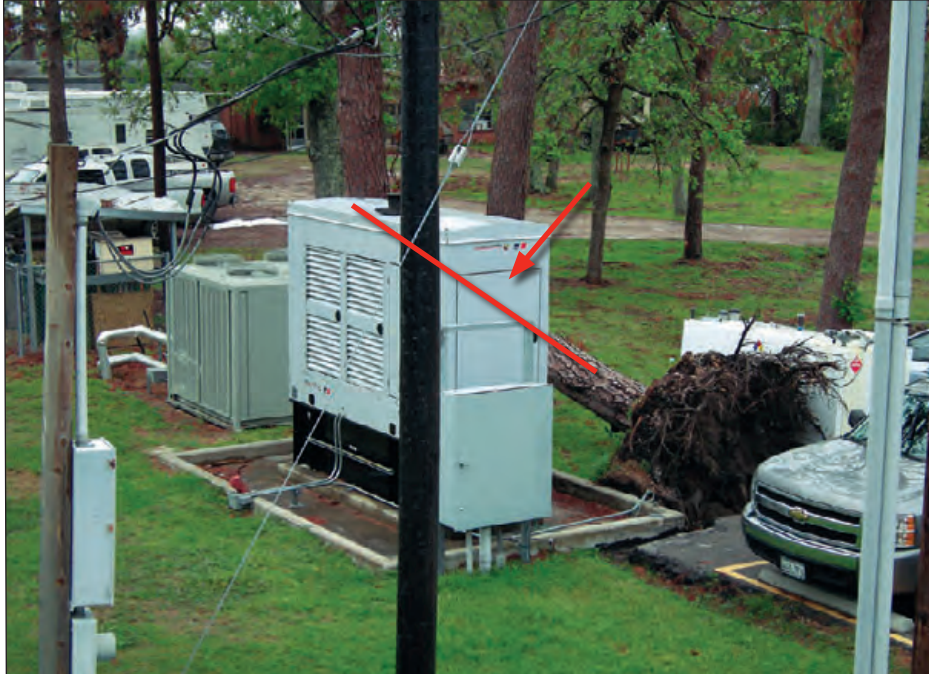
Figure 6-119: The tree shown by the red line nearly fell on the emergency generator (red arrow). Estimated wind speed: 110 mph. Hurricane Ike (Texas, 2008)
