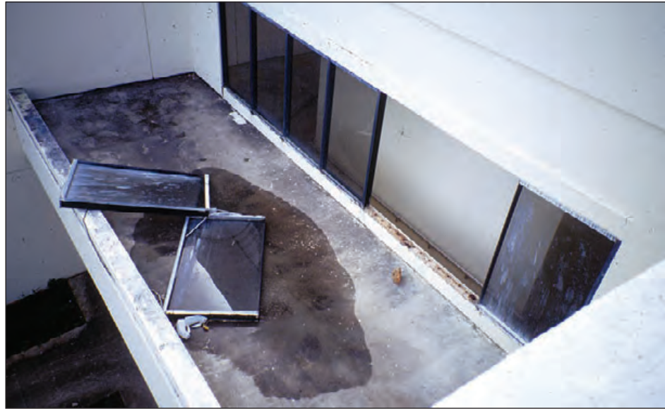
Figure 6-50: Two complete windows, including frames, blew out as a result of an inadequate number of fasteners. Typhoon Paka (Guam, 1997)
