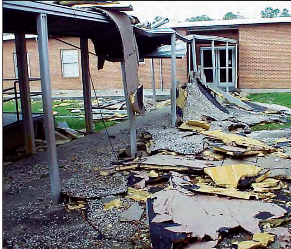
Figure 6:33: Open walkways do not provide protection from wind-borne debris. Hurricane Katrina (Mississippi, 2005).
