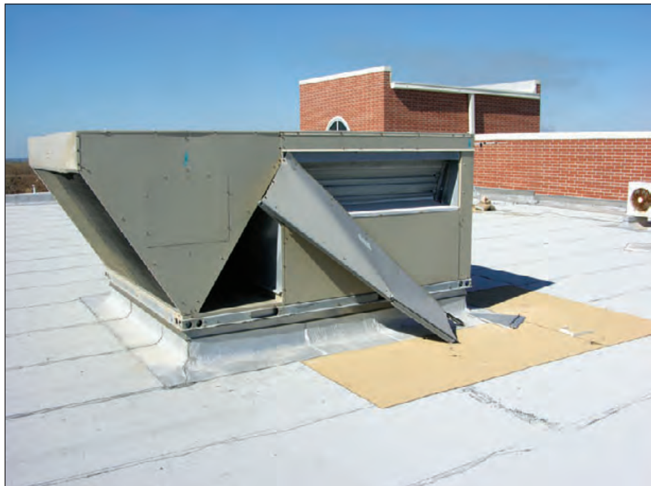
Figure 6-136: At this school, the hood on this HVAC unit was inadequately attached. A strap between the hood and unit can be economically installed to avoid this problem. Estimated wind speed: 110 mph. Hurricane Ike (Texas, 2008)
