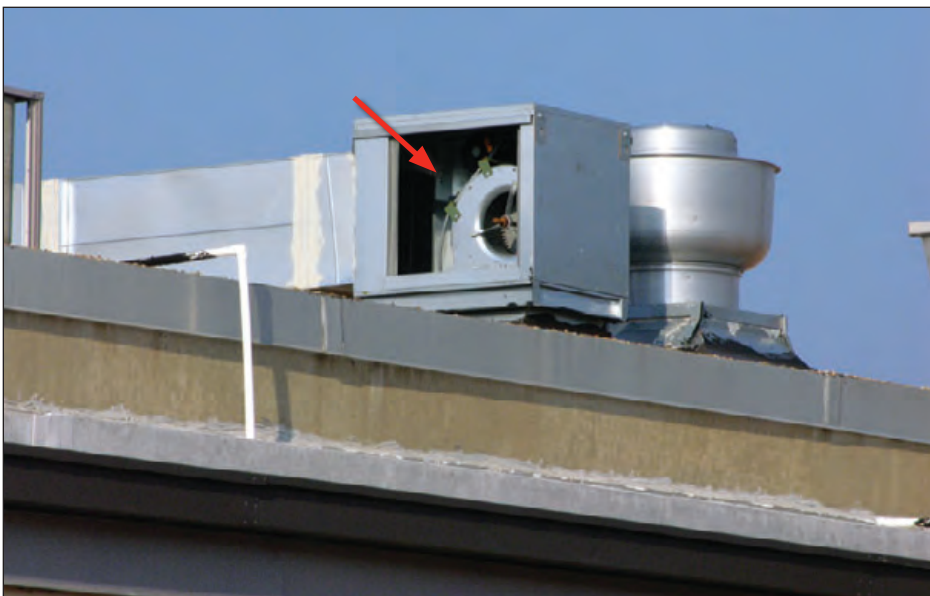
Figure 6-98: The school shown in Figure 6-65 also had an access panel blow off. Blown-off panels can puncture roof membranes, break glazing, and cause injury. Estimated wind speed: 85–95 mph. Hurricane Ivan (Florida, 2004)
