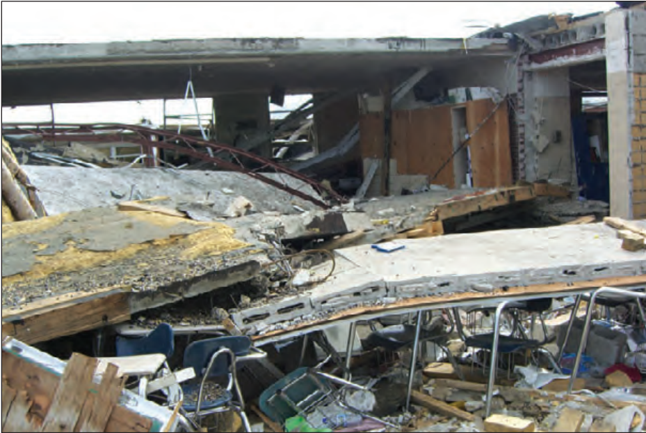
Figure 6-143 : Unreinforced masonry walls and hollow-core concrete roof planks collapsed. Enterprise Tornado (Alabama, 2007)
