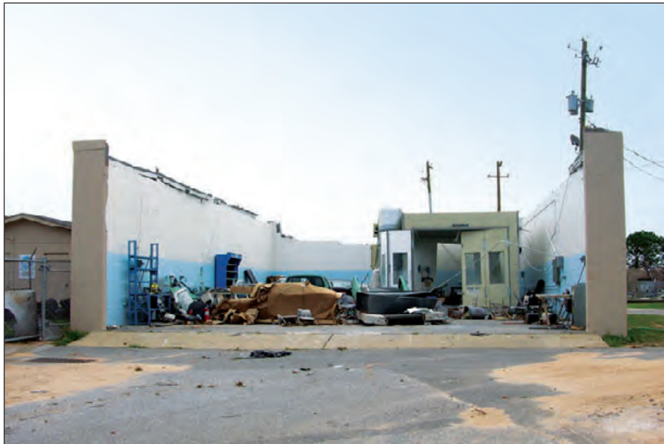
Figure 6-21: The entire metal deck and steel joist roof structure at this school's auto shop blew off. Estimated wind speed: 105 to 115 mph. Hurricane Ivan (Florida, 2004)
