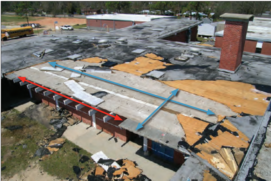
Figure 6-121 The cementitious wood-fiber deck panels blew off of much of the overhang at this school. Deck panel failure resulted in lifting and peeling of the roof system over a large area, exposure of the decking in the area shown by the blue arrows, and extensive interior water infiltration. Estimated wind speed: 105–115 mph. Hurricane Ivan (Florida, 2004)
