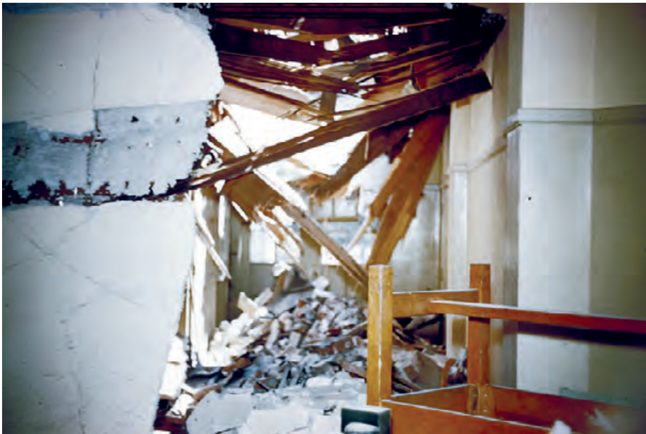
Figure 4-17: Destroyed exit corridor, Bakersfield, Kern County, CA, 1952
