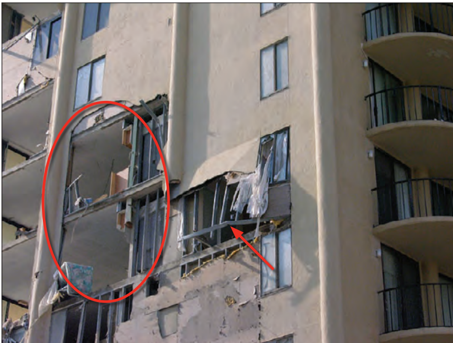
Figure 6-63: The stucco wall failure was caused by inadequate attachment between the stud tracks and the building's structure. All of the metal stud framing within the red oval blew away. The arrow shows a bottom stud track that detached and pulled away from the building. Estimated wind speed: 110–125 mph. Hurricane Ivan (Florida, 2004)
