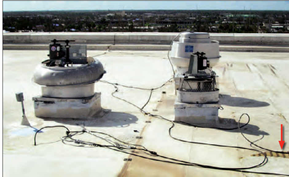
Figure 6-92: Cowlings blew off two of the three fans. Note also the loose LPS conductors and missing walkway pad (red arrow). Estimated wind speed: 140–160 mph. Hurricane Charley (Florida, 2004)
