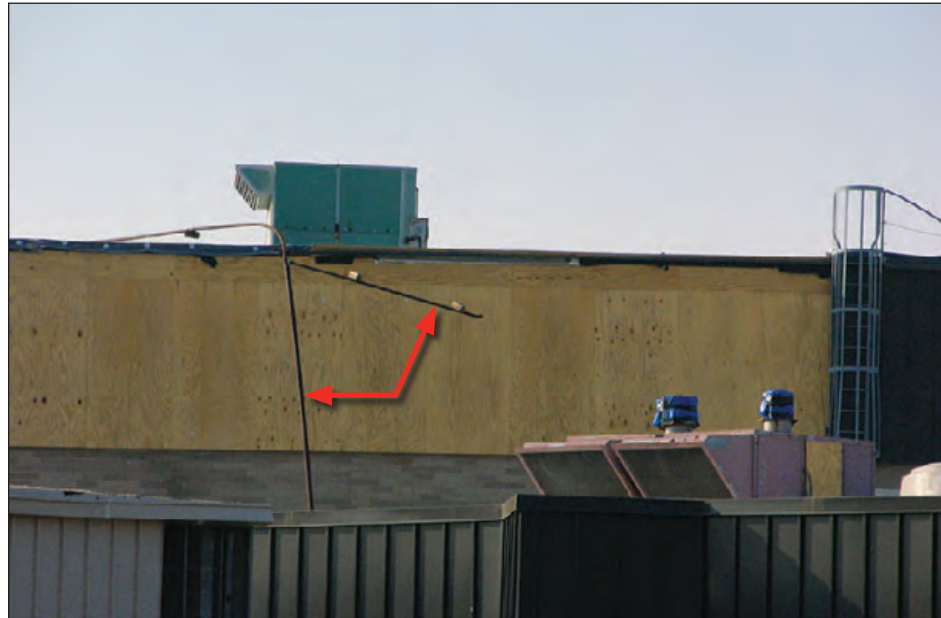
Figure 6-99: The school shown in Figures 6-65 and 6-98 also experienced gas line rupture (shown by the lines dangling over the side of the building). Estimated wind speed: 85–95 mph. Hurricane Ivan (Florida, 2004)
