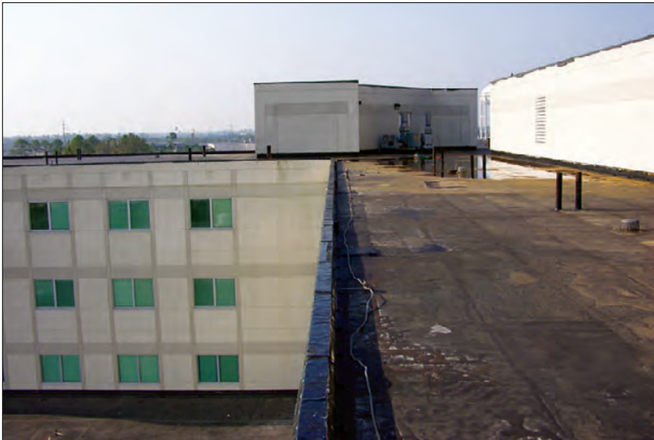
Figure 6-120: The roof and a portion of the EIFS on this 5-year-old building blew off. Water leaked into the floor below. The floor was taken out of service for more than a month. Estimated wind speed: 130 mph. Hurricane Katrina (Mississippi, 2005)
