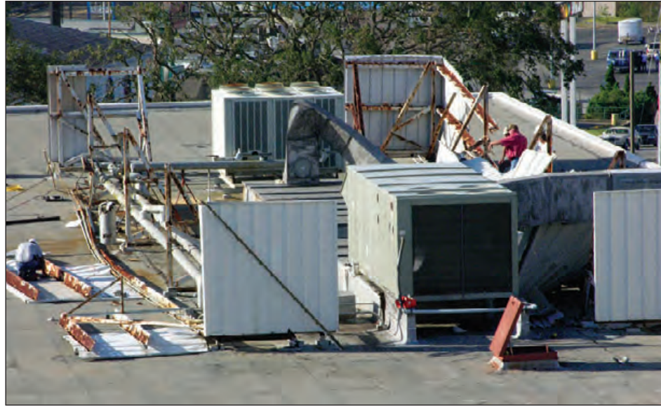
Figure 6-102: Equipment screen panels can puncture roof membranes, break glazing, and cause injury. Estimated wind speed: 105–115 mph. Hurricane Ivan (Florida, 2004)
