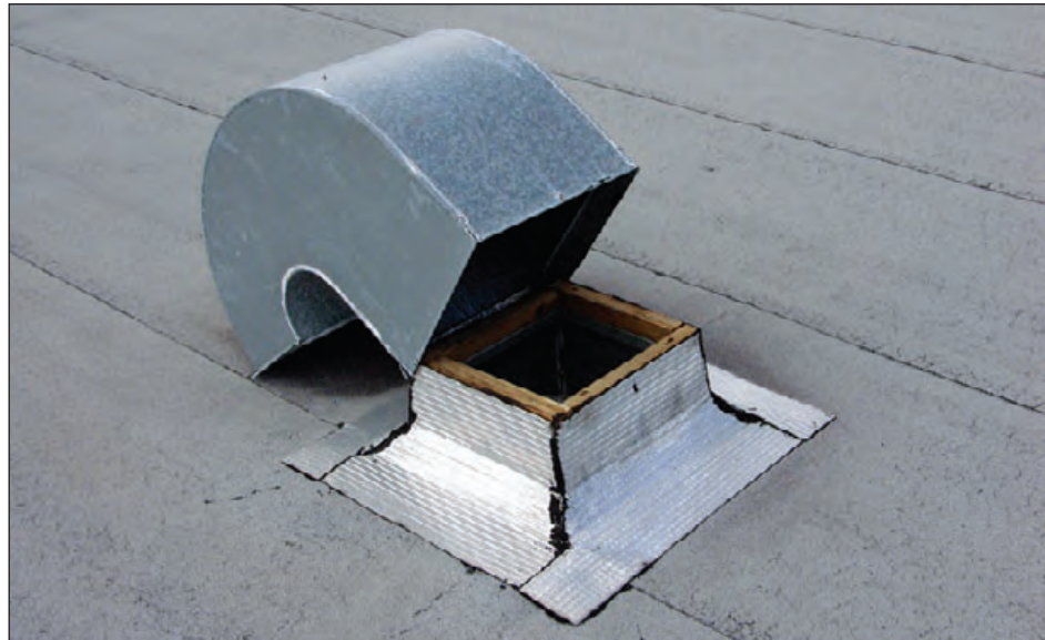
Figure 6-89: This gooseneck was attached with only two small screws. Emergency repairs had not been made at the time this photograph was taken, which was 5 days after the hurricane struck. A substantial amount of water was able to enter the school. Hurricane Francis (Florida, 2004)
