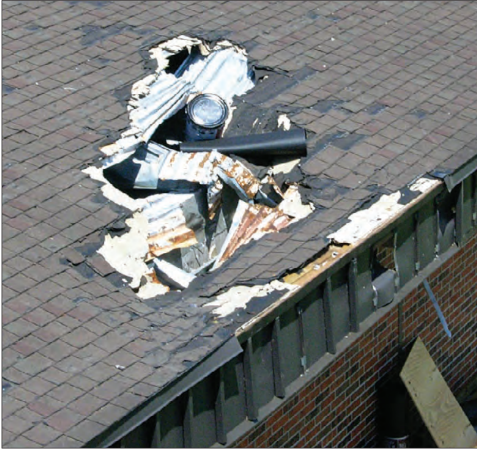
Figure 6-42: At the school shown in Figure 6-34, wind-borne debris ruptured the proprietary composite deck system composed of light gauge corrugated metal deck and gypsum board. Estimated wind speed: 140 to 160 mph. Hurricane Charley (Florida, 2004)
