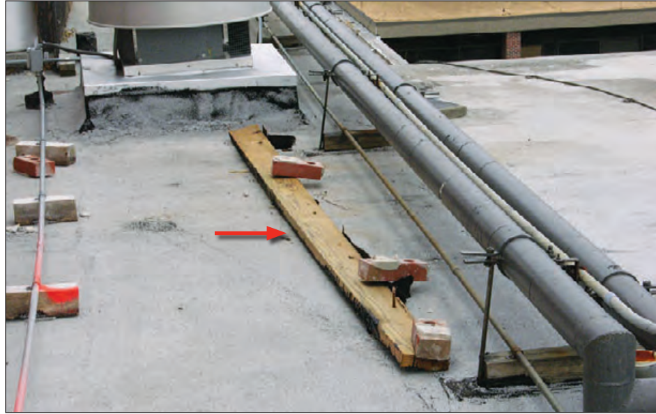
Figure 6-132: The nailer (red arrow) blew off an upper roof and landed on the roof below. The nailer was anchored to a brick wall. Some of the anchors pulled out of the brick, and some of the bricks blew away with the nailer. Estimated wind speed: 105–115 mph. Hurricane Ivan (Florida), 2004
