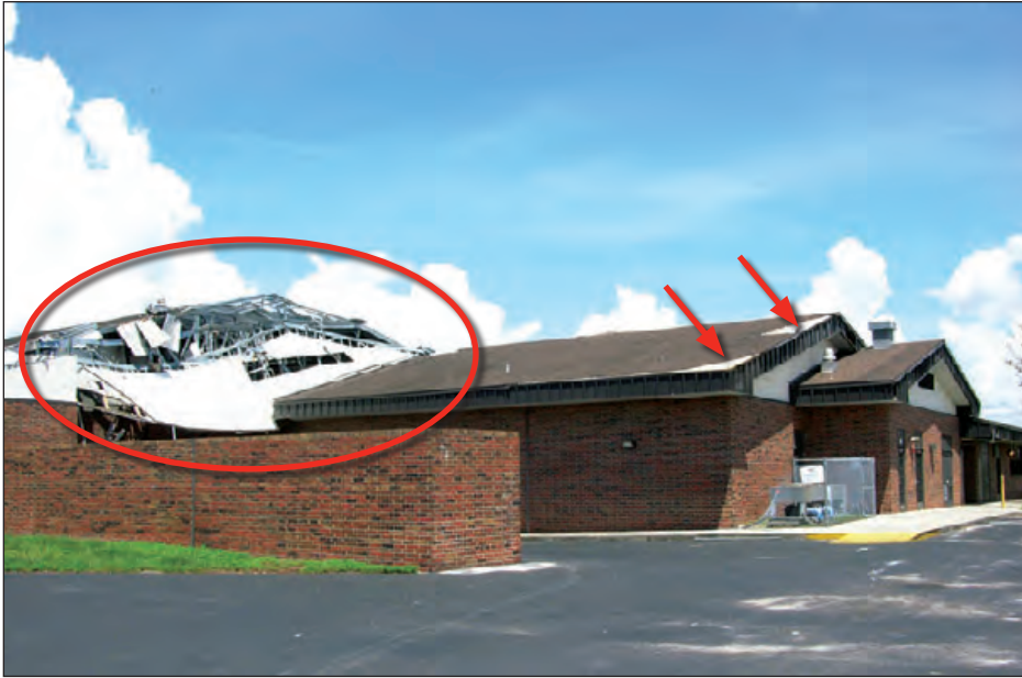
Figure 6-34: The structure on this school was composed of light gauge metal framing, with a proprietary composite deck system composed of light gauge corrugated metal deck and gypsum board. In addition to the gable end wall failure, the asphalt shingles and underlayment were blown off at the corner of the eave and ridge. Estimated wind speed: 140 to 160 mph. Hurricane Charley (Florida, 2004)
