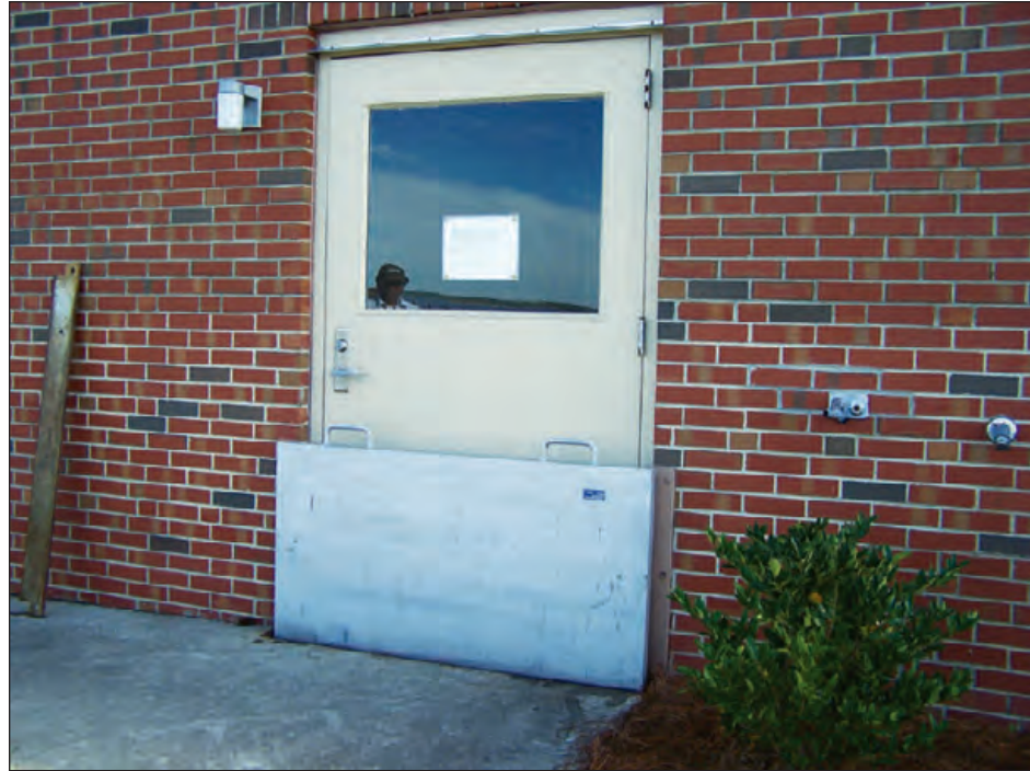
Figure 5-26: Specially designed panels are mounted to block doors, windows, and other openings to keep water from entering the building.
