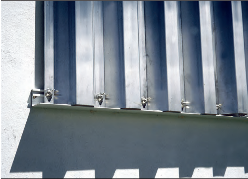
Figure 6-126: A metal panel shutter. Hurricane Georges (Puerto Rico, 1998)
