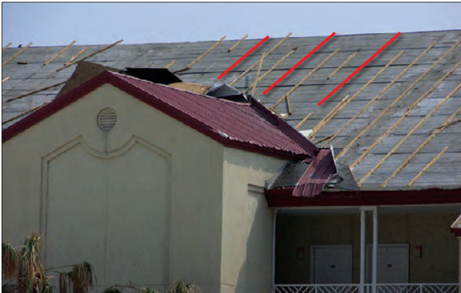
Figure 6-30: In most of the areas on this roof, the connection of the top nailer to the bottom nailer was the weakest link. However, in a few locations, the connection of the bottom nailer to the roof structure was the weak link (three of the blown-off bottom nailers are shown by the red lines).
