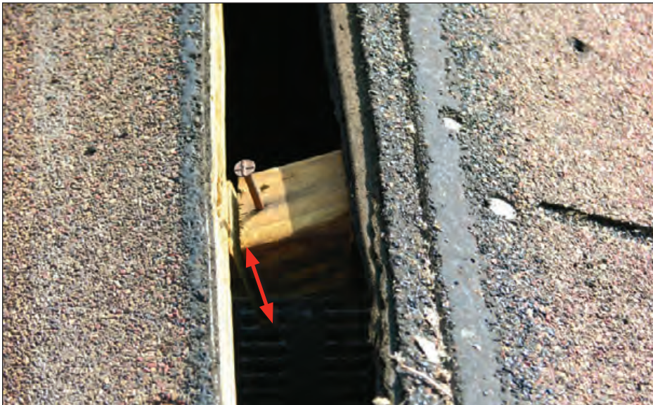
Figure 6-134: During a reroofing project a slot was cut in the plywood deck in order to allow air to flow from the attic to a new continuous ridge vent. The cutting depth of the saw was not adjusted for the thickness of the deck. The top 1½ inch of each truss and a portion of the metal nailing plate was inadvertently cut.
