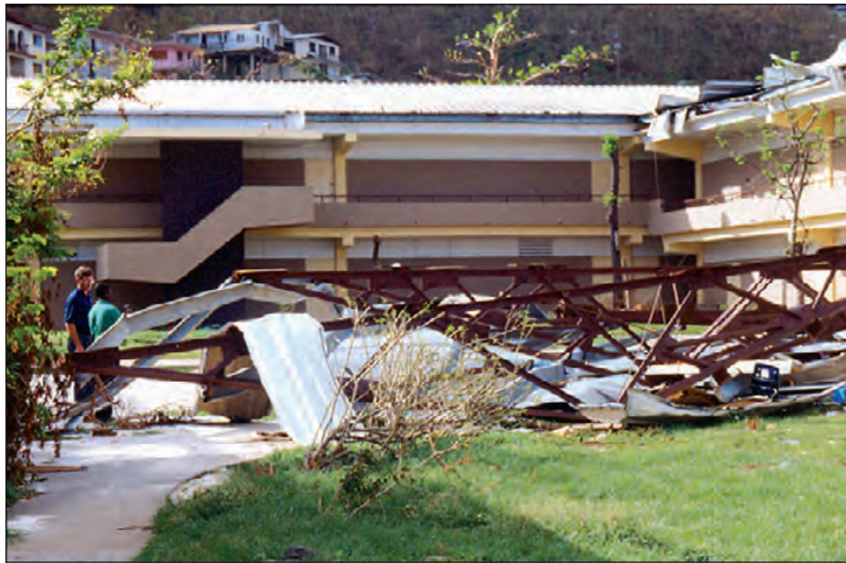
Figure 6-122: The steel truss superstructure installed on this school as part of a steep-slope conversion blew away because of inadequate attachment. Hurricane Marilyn (U.S. Virgin Islands, 1995)
