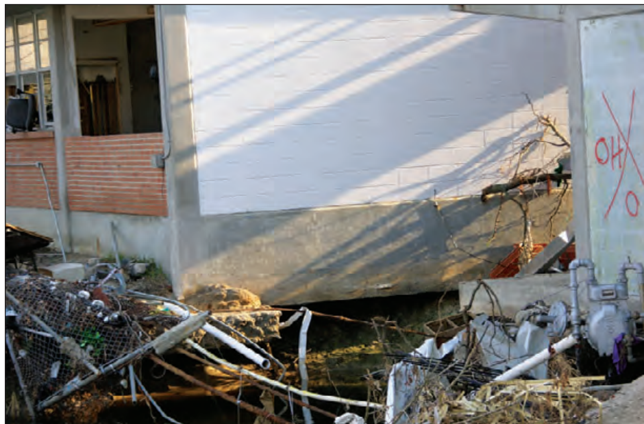
Figure 5-16: Scour undermined the foundation of St. Paul Catholic School, Pass Christian, LA.
