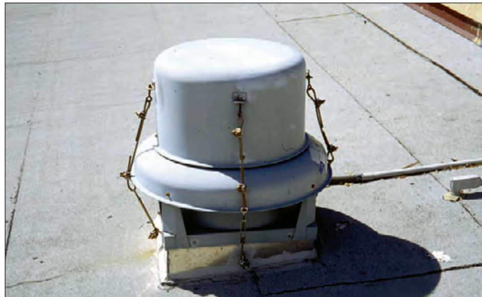
Figure 6-93: Cables were attached to prevent the cowling from blowing off. Typhoon Paka (Guam, 1997)
