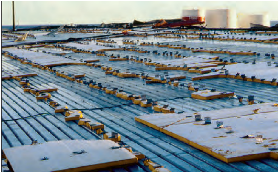
Figure 6-82: Significant interior water damage and facility interruption occurred after the standing seam roof blew off. Hurricane Marilyn (U.S. Virgin Islands, 1995)
