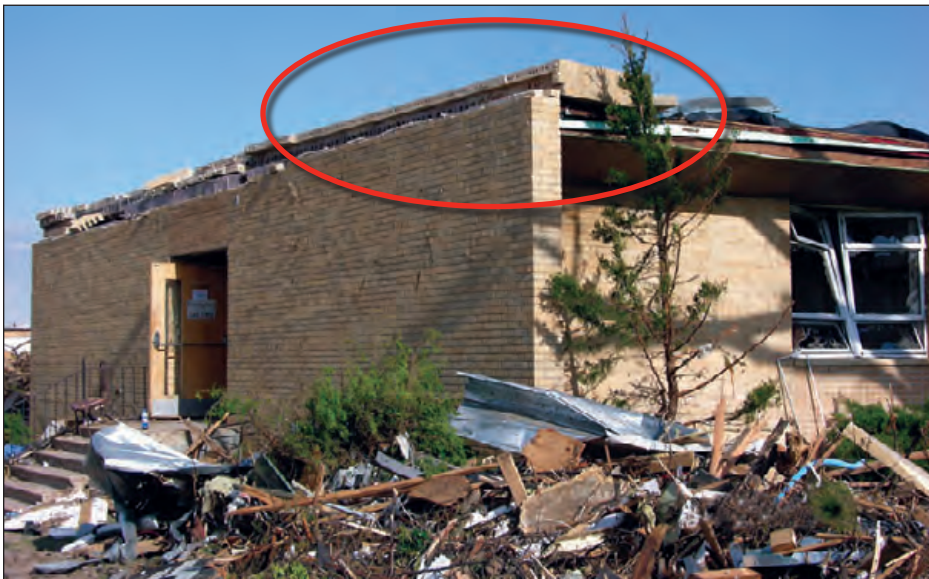
Figure 6-129: Collapsed unreinforced masonry parapet. Greensburg Tornado (Kansas, 2007)
