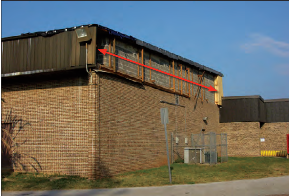
Figure 6-65: Blow-off of metal fascia panels due to inadequate attachment of wood furring to the CMU wall. Estimated wind speed: 85–95 mph. Hurricane Ivan (Florida, 2004)
