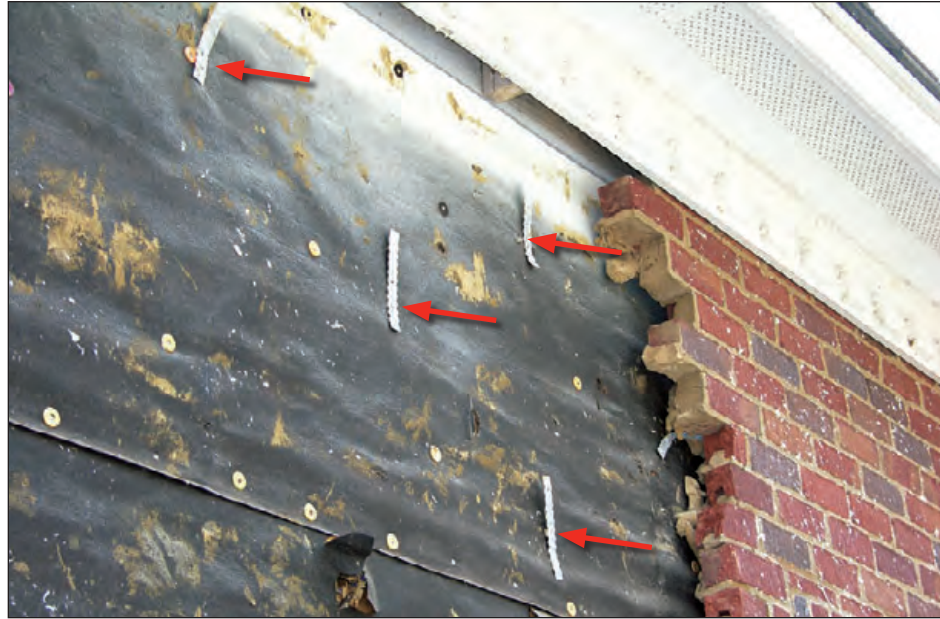
Figure 6-58: The four ties shown by the red arrows were not embedded into the mortar. Estimated wind speed: 105 mph. Hurricane Katrina, (Mississippi, 2005)
