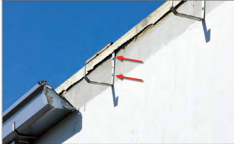
Figure 6-74: Because this gutter was not attached to the bracket, wind lifted the gutter along with the metal edge flashing that lapped into the gutter. Bracket fasteners are indicated by the red arrows. Hurricane Francis (Florida, 2004)
