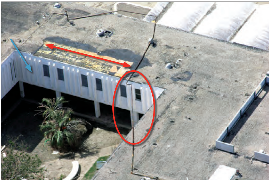
Figure 6-57: Although uncommon for schools, precast wall panels were attached to the structural frame of this school. This type of wall typically offers excellent wind performance. Note the roof covering damage and displaced gas line. Estimated wind speed: Approximately 125–130 mph. Hurricane Katrina (Louisiana, 2005)
