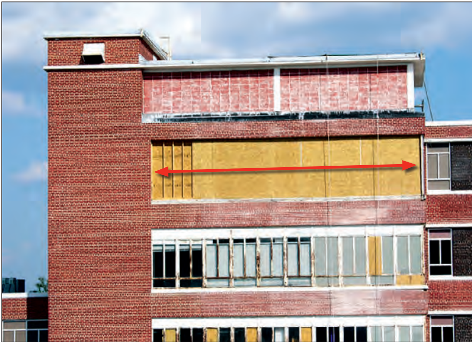
Figure 6-123: Wind pressure caused the window frames on the upper floors to fail (red arrow). Estimated wind speed: 130 mph. Hurricane Katrina (Mississippi, 2005)
