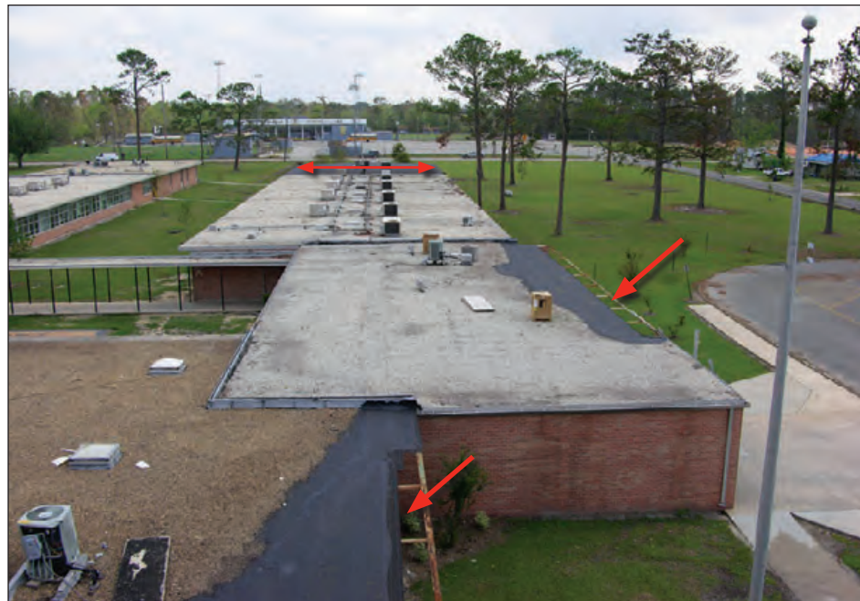
Figure 6-26: The cementitious wood-fiber deck panels blew off the overhangs and caused a progressive lifting and peeling of the roof membrane. Strengthening (or replacing) inadequately attached roof decks during a reroofing project is both prudent and relatively economical. Estimated wind speed: 120 mph. Hurricane Katrina (Mississippi, 2005)
