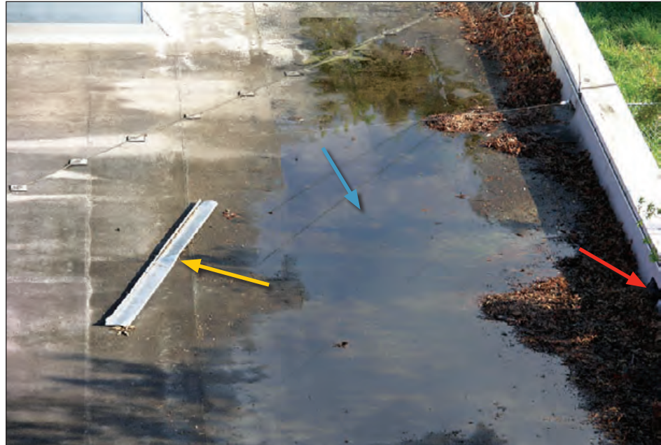
Figure 6-104: Leaf debris and ponding near a scupper (red and blue arrows). The yellow arrow indicates a piece of coping that blew off an upper roof shown in Figure 6-72. Estimated wind speed: 92 mph. Hurricane Ike (Texas, 2008)
