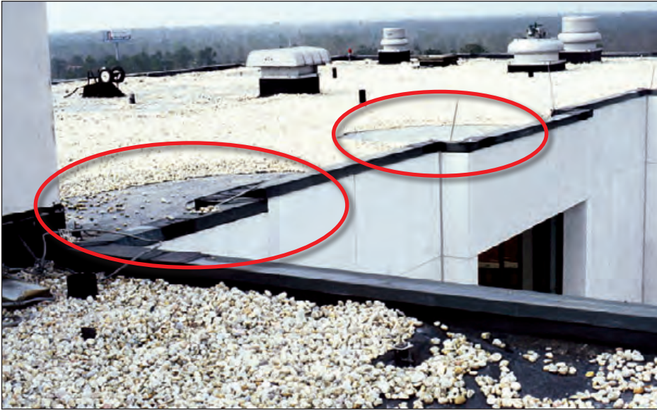
Figure 6-8: Aggregate blow-off associated with building irregularities. Hurricane Hugo (South Carolina, 1989)
