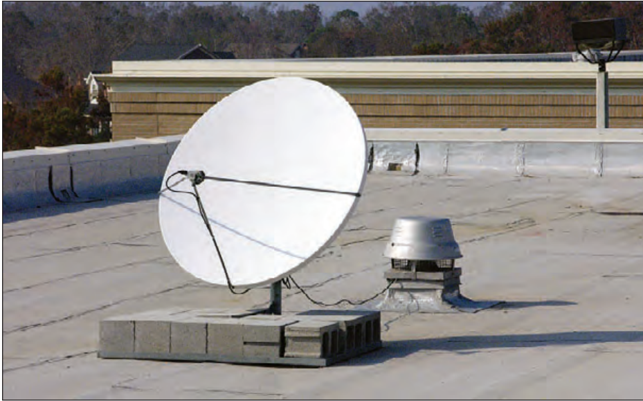
Figure 6-107: Common anchoring method for satellite dish. Estimated wind speed: 85–95 mph. Hurricane Ivan (Florida, 2004)
