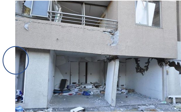
Figure 3.5-2 A change in the wall section from the upper to lower story (circled) results in a loss of wall area and localization of flexural yielding (Plaza del Rio Building, Concepcion, Chile)
