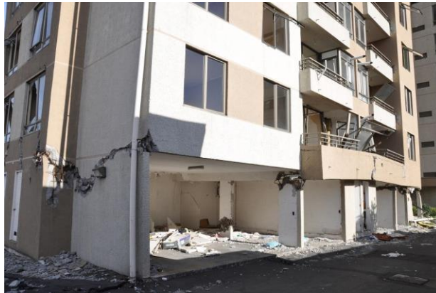
Figure 3.5-1 Coupled walls in upper stories do not continue to lower story (Plaza del Rio Building, Concepcion, Chile)
