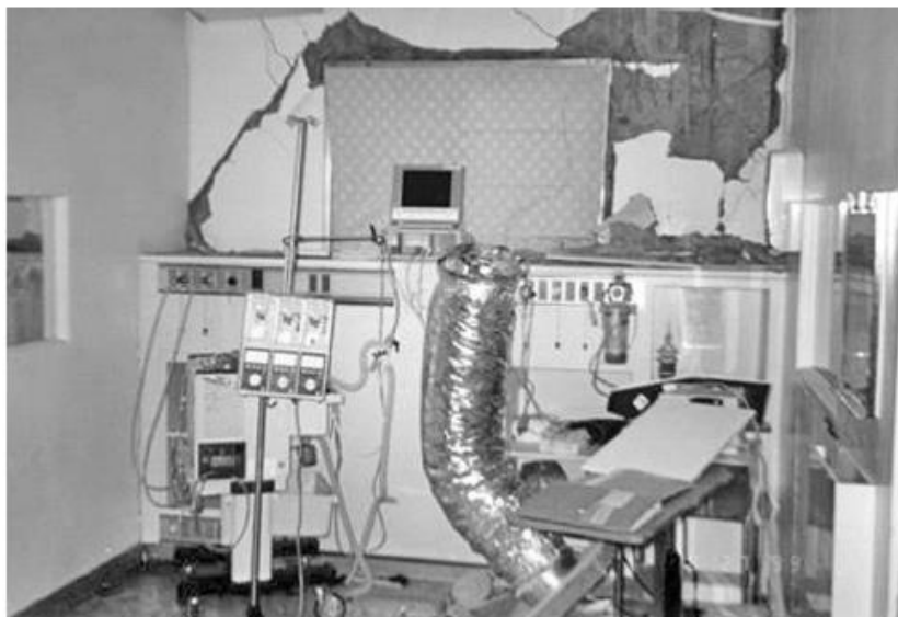
FIGURE C13.1-6 Collapsed Duct and HVAC Diffuser
