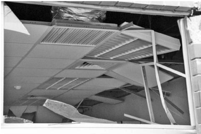
FIGURE C13.1-2 Damaged Ceiling System
