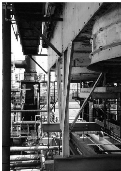
FIGURE C13.6-1 Fin Fan Elevated on Integral Supports
